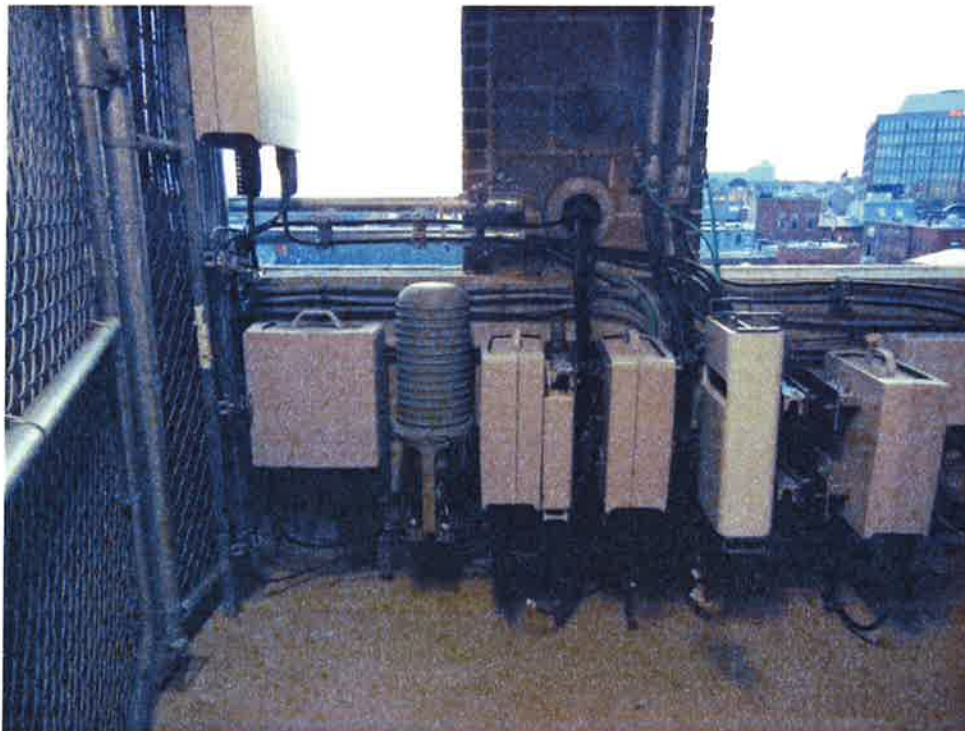
Photo 4: Sample photo illustrating the existing RRH's and surge arrestor.
