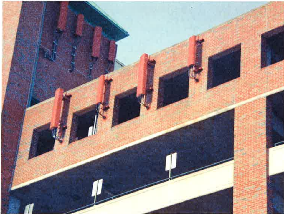
Photo 3: Sample photo illustrating the existing Gamma sector antennas.
