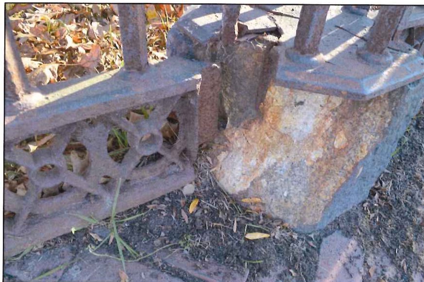
TYPICAL DAMAGED FENCE POST - CUT REPLACEMENT
