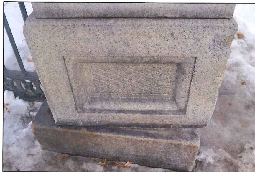
OUT OF SQUARE & PLUMB - REALIGN
