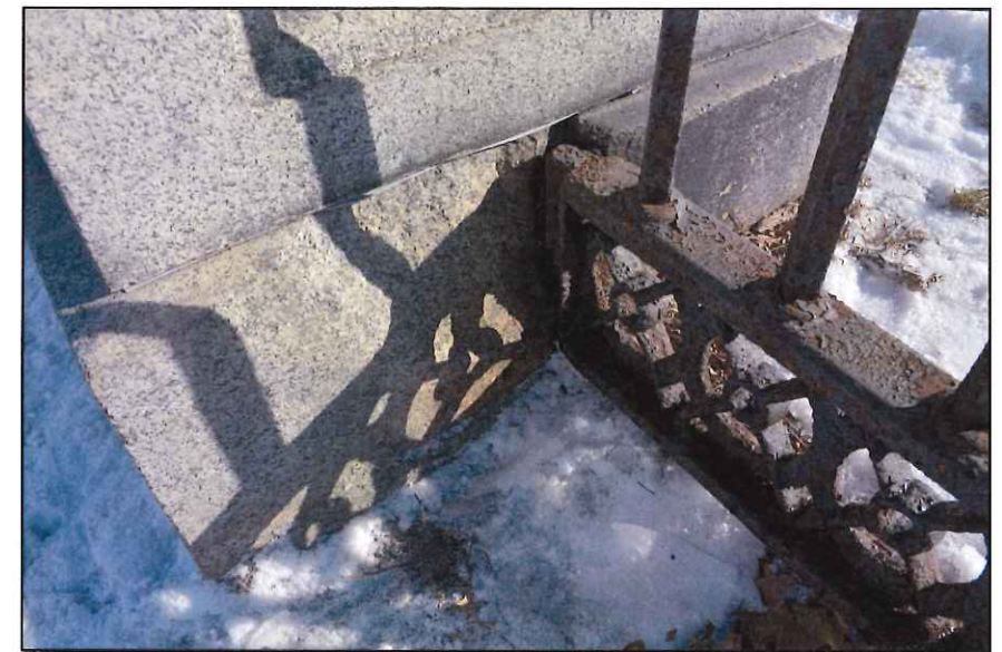
TYPICAL DAMAGED GRANITE - SECTION REPAIR
