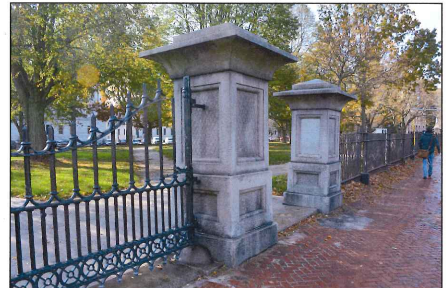
MISSING GATE PIECES - RECAST REPLACEMENTS
