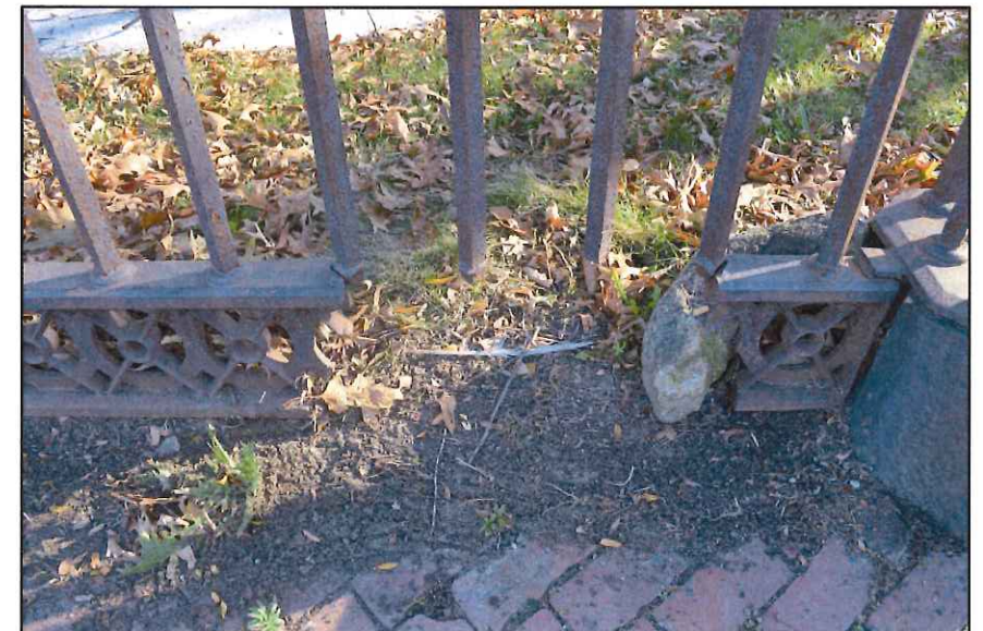
MISSING BOTTOM RAIL SECTION - RECAST REPLACEMENT
