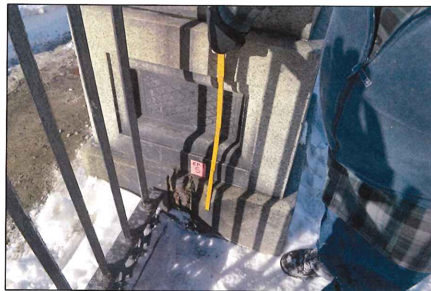
PAINT & RUST STAINING - CLEANING
