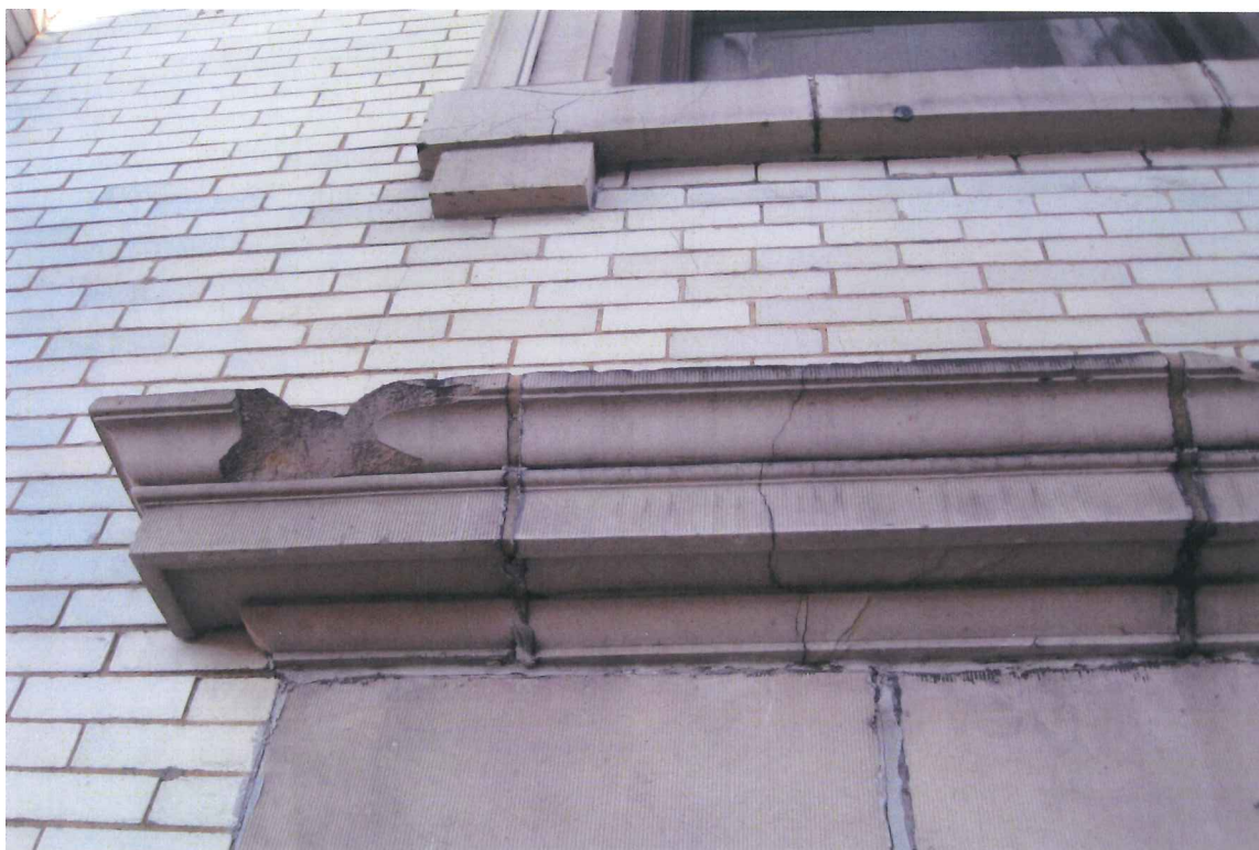
Photo 6: Netting was not installed over all projecting terra cotta units. Structures North, 2009.
