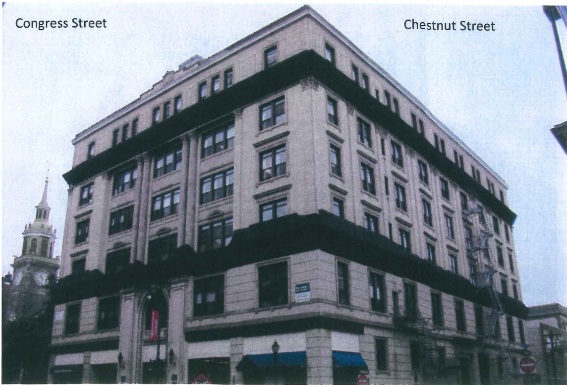
Photo 2: 415 Congress Street is a brick building with terra cotta trim. The netting on the upper and lower cornices was installed approximately three years ago. SCC, June 2009.
