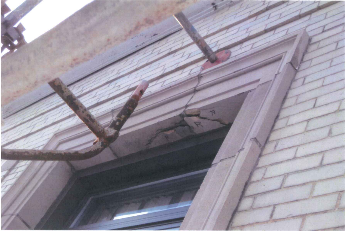
Photo 11: Cracking and spalling of window lintel soffits. Structures North, Dec 2009.
