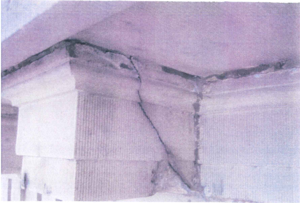
Photo 9: Detail of cracked block modillion at cornice. Structures North, Dec 2009.
