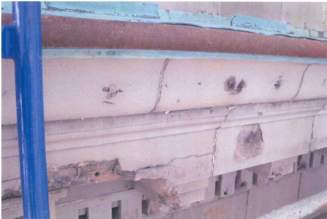
Photo 8: Detail of typical conditions at cornice. Structures North, Dec 2009.
