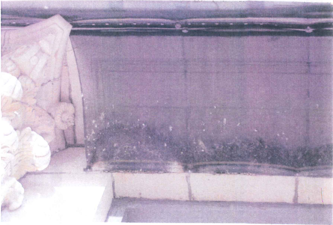
Photo 5: Netting at cornices has collected pigeon guano. Structures North, Dec 2009.
