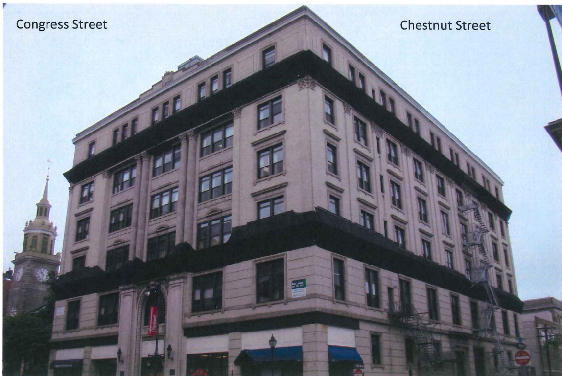
Photo 2: 415 Congress Street is a brick building with terra cotta trim. The netting on the upper and lower cornices was installed approximately three years ago. SCC, June 2009.
