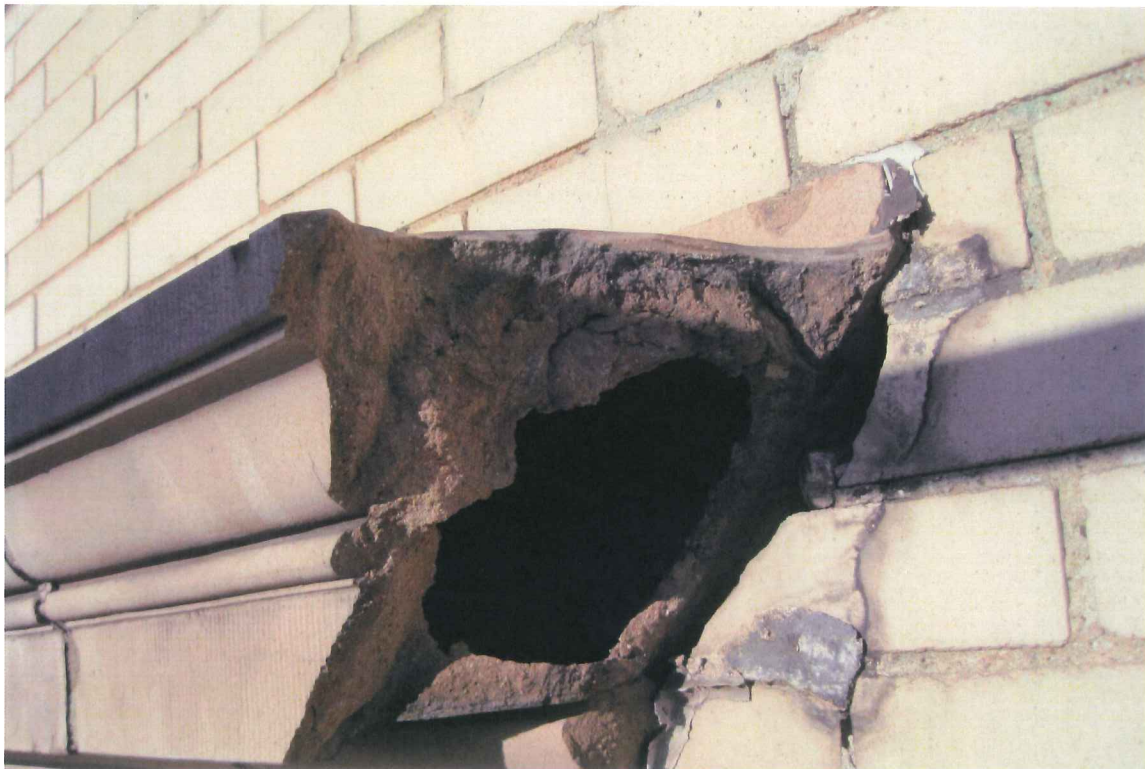
Photo 4: Detail of terra cotta window head at missing piece. Structures North Consulting Engineers (Structures North), Dec 2009.
