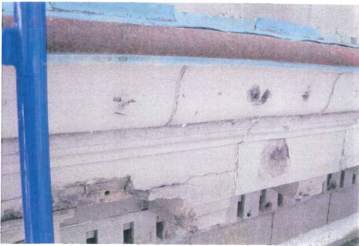
Photo 8: Detail of typical conditions at cornice. Structures North, Dec 2009.
