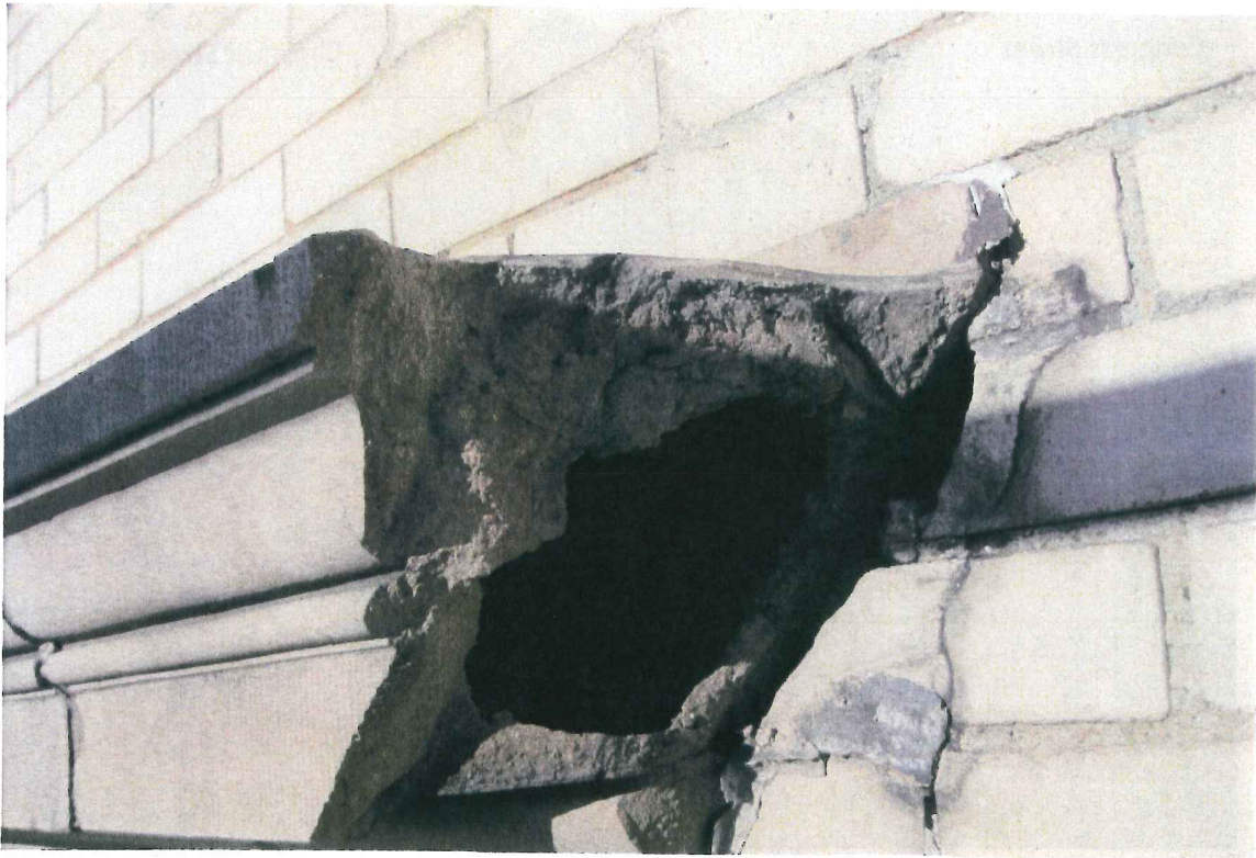
Photo 4: Detail of terra cotta window head at missing piece. Structures North Consulting Engineers (Structures North), Dec 2009.
