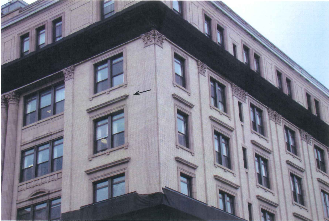
Photo 3: In June 2009 a piece of terra cotta from a 4th floor projecting window head fell from the building. SCC, June 2009.
