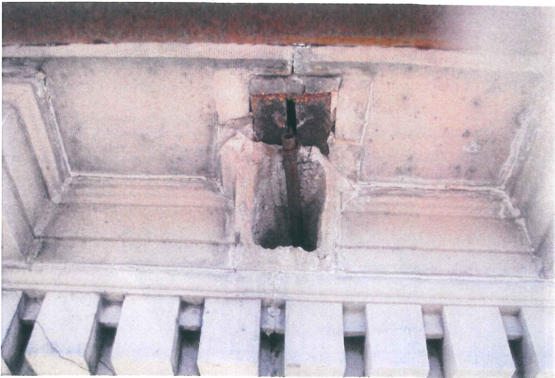
Photo 10: Detail of steel armature after removal of broken block modillion. Note cracked dentils below. Structures North, Dec 2009.
