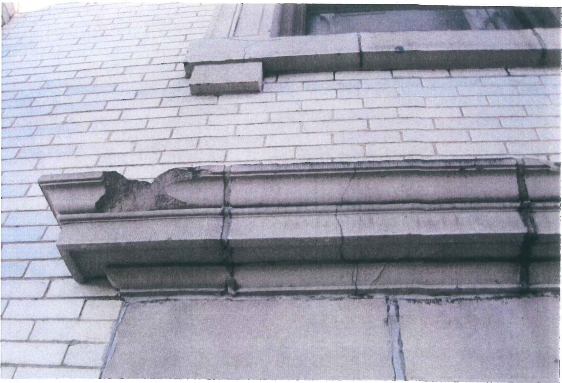
Photo 6: Netting was not installed over all projecting terra cotta units. Structures North, 2009.
