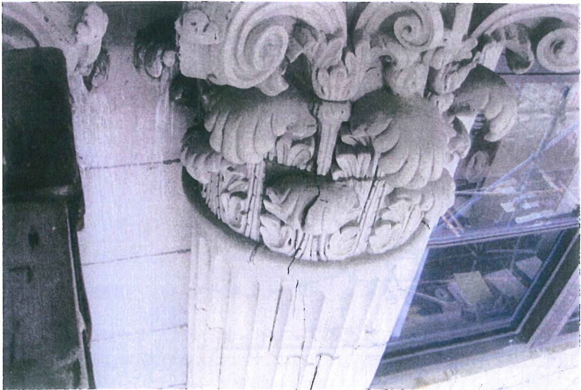
Photo 14: Detail of column and capital on Congress Street facade. Structures North, Dec 2009.
