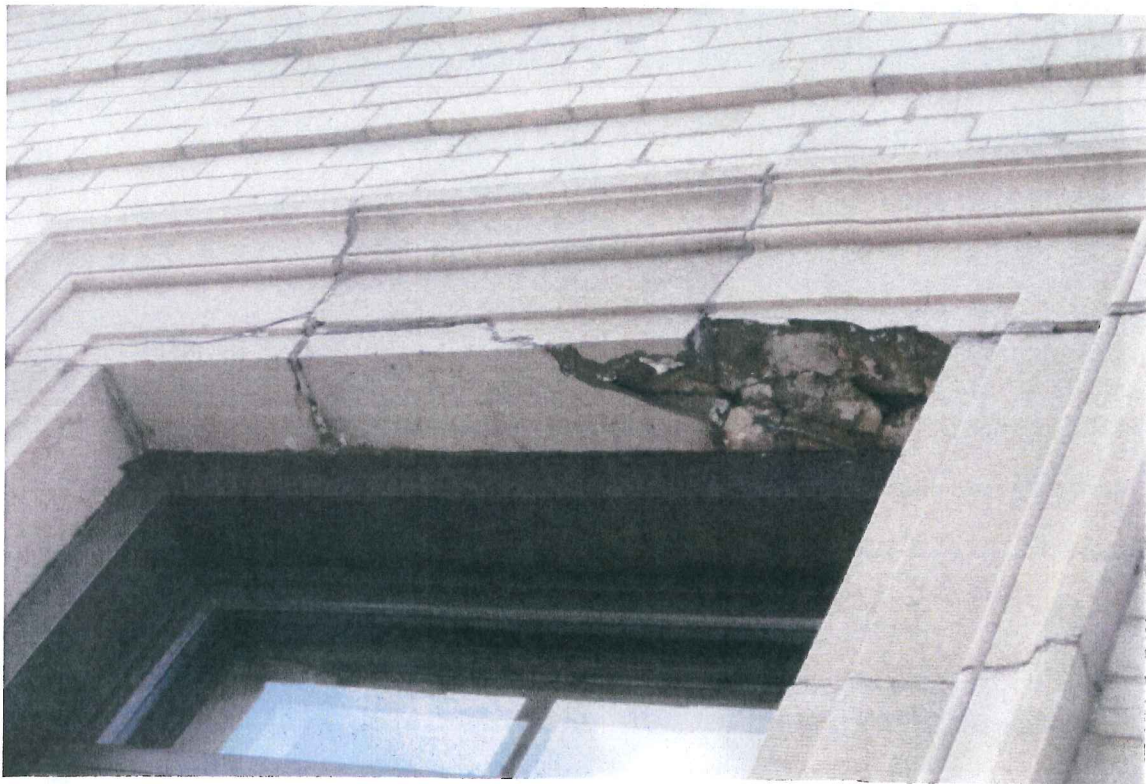
Photo 12: Cracking and spalling of window lintel soffits. Structures North, Dec 2009.
