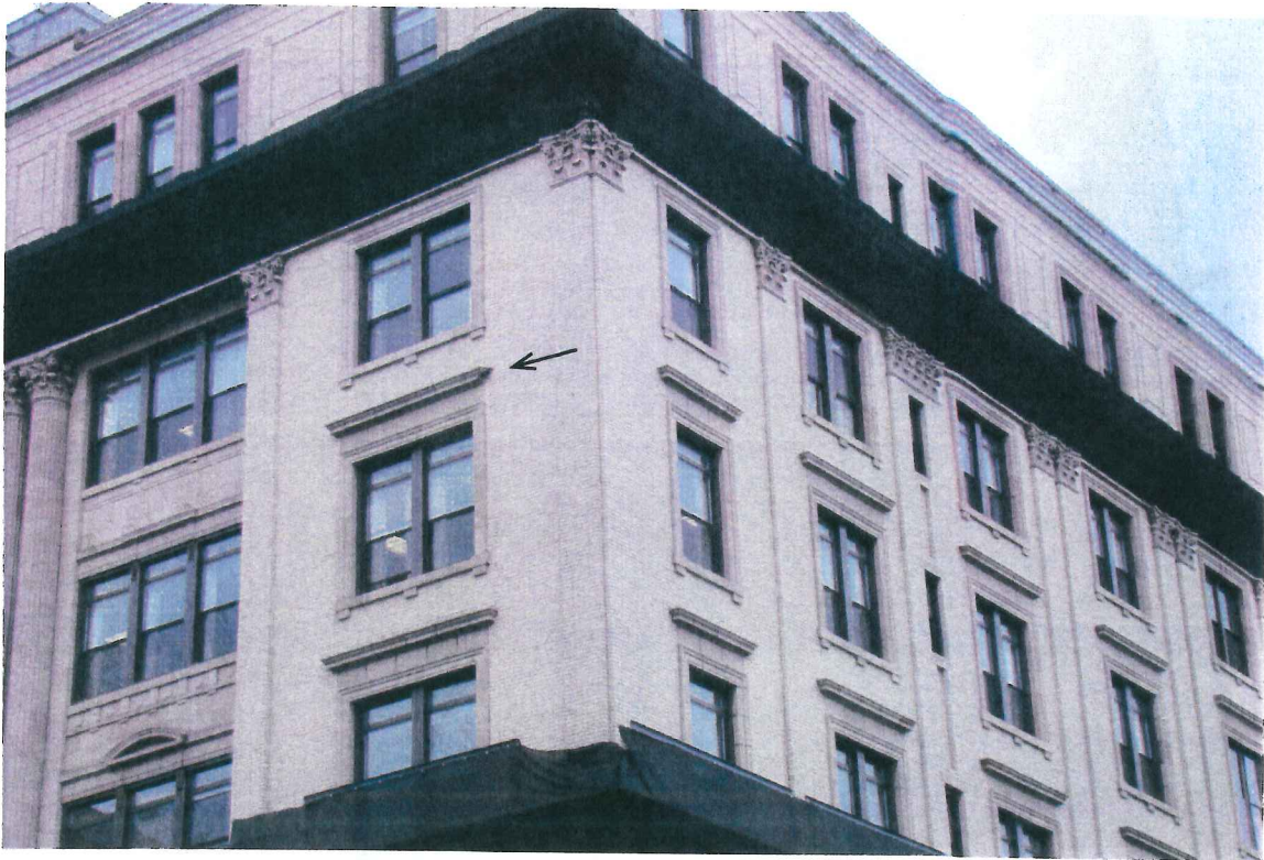
Photo 3: In June 2009 a piece of terra cotta from a 4th floor projecting window head fell from the building. SCC, June 2009.
