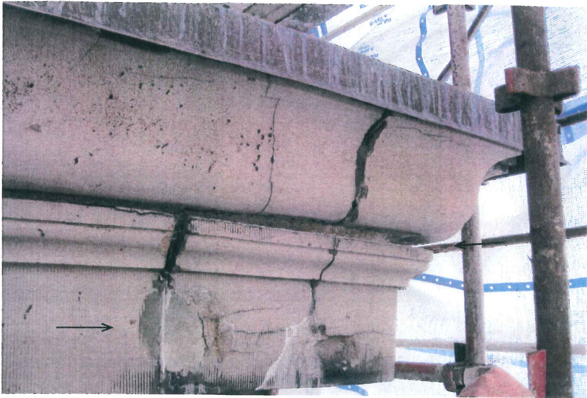
Photo 7: Detail of corner cornice units to be removed. Note earlier cementitious patching repair. Structures North, Dec 2009.
