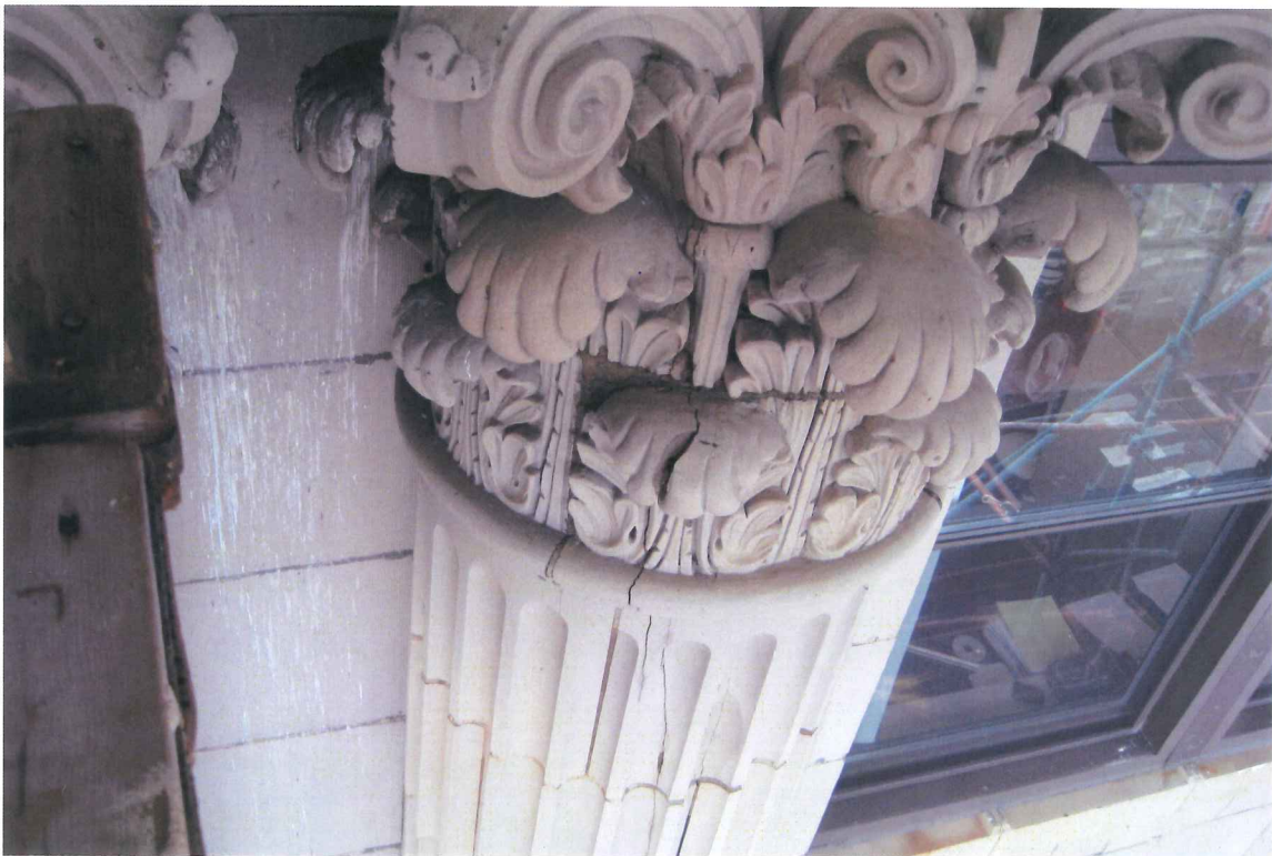
Photo 14: Detail of column and capital on Congress Street facade. Structures North, Dec 2009.
