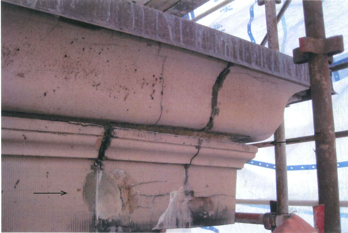
Photo 7: Detail of corner cornice units to be removed. Note earlier cementitious patching repair. Structures North, Dec 2009.
