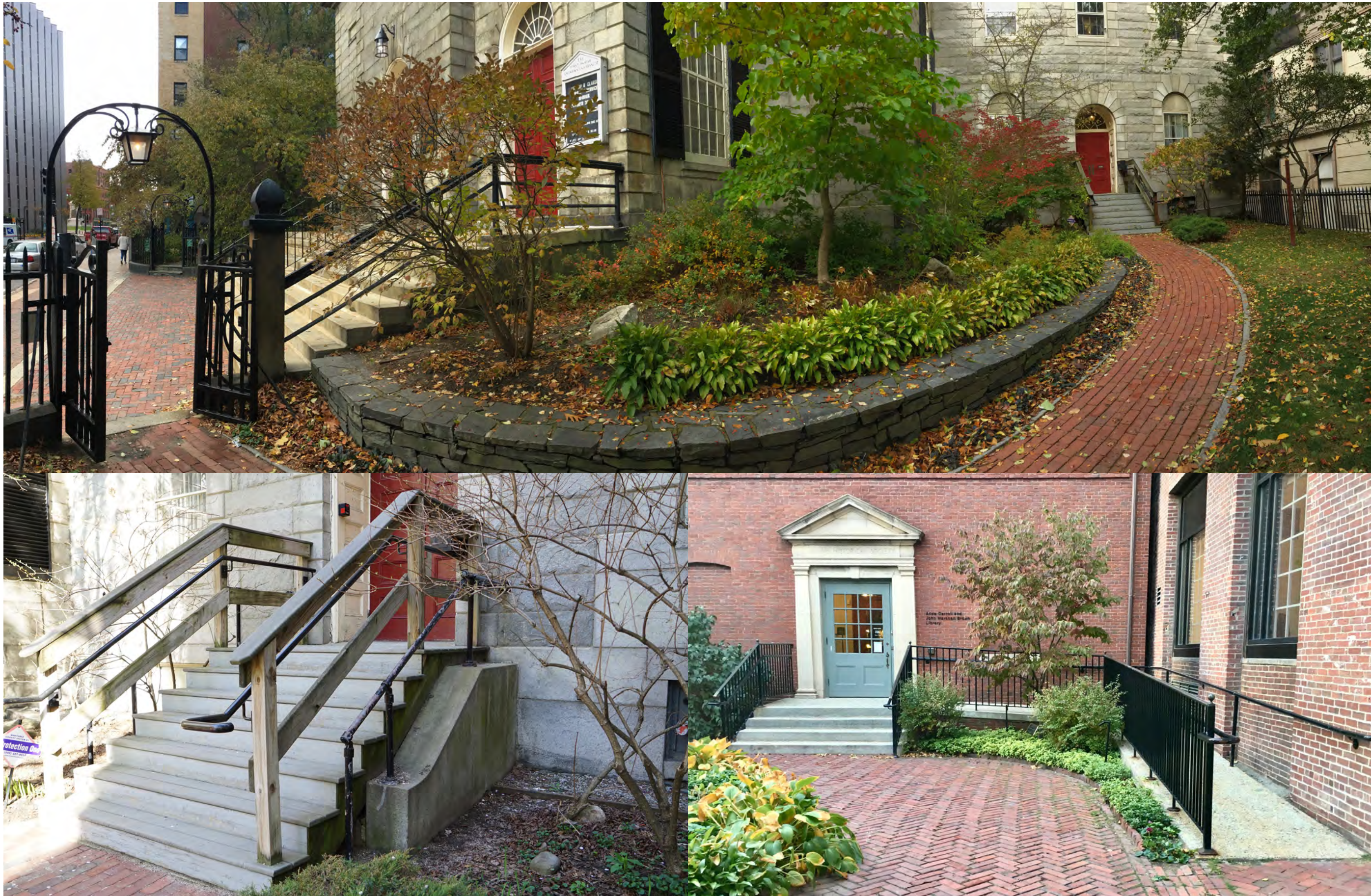
Top: Parish House Garden and Front entry stairs. Bottom Left: Original granite stairs with current overlay stairs, landing and handrails. Bottom Right: Maine Historical Society's painted steel guard and handrail system.
