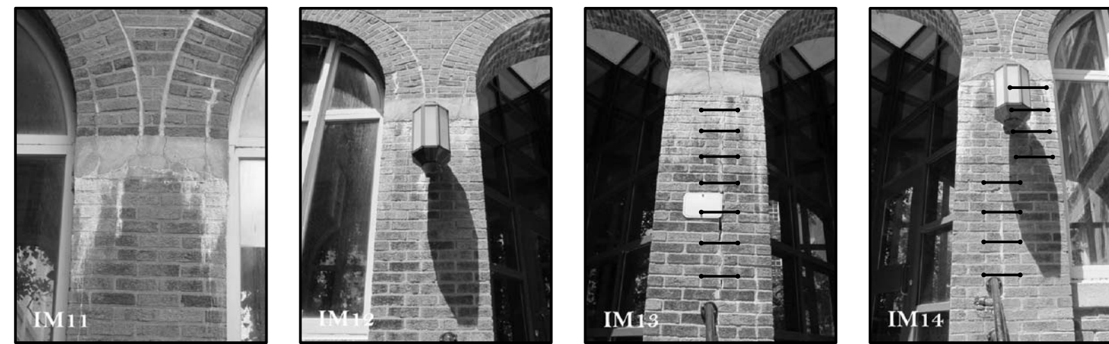
T03A SPRING BLOCK: REPLACE W/ GRANITE VENEER. CLEAN BRICK T03B SPRING BLOCK: REPLACE W/ GRANITE VENEER. CLEAN BRICK T03C SPRING BLOCK: REPLACE W/ GRANITE VENEER. CLEAN AND REPAIR BRICK. SEE DETAIL 10/A-22 T03D SPRING BLOCK: REPLACE W/ GRANITE VENEER. CLEAN AND REPAIR BRICK. SEE DETAIL 10/A-22
