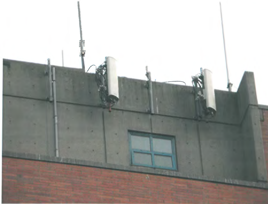
Photo 3: Sample photo illustrating the existing Gamma sector antennas.
