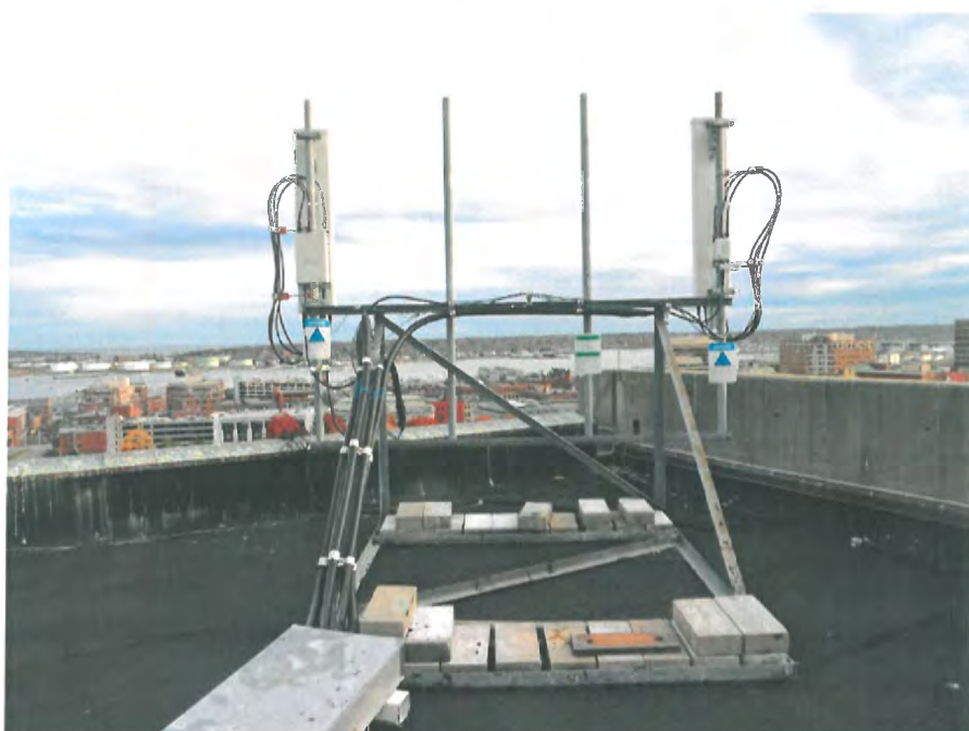
Photo 2: Sample photo illustrating the existing Beta sector antennas.
