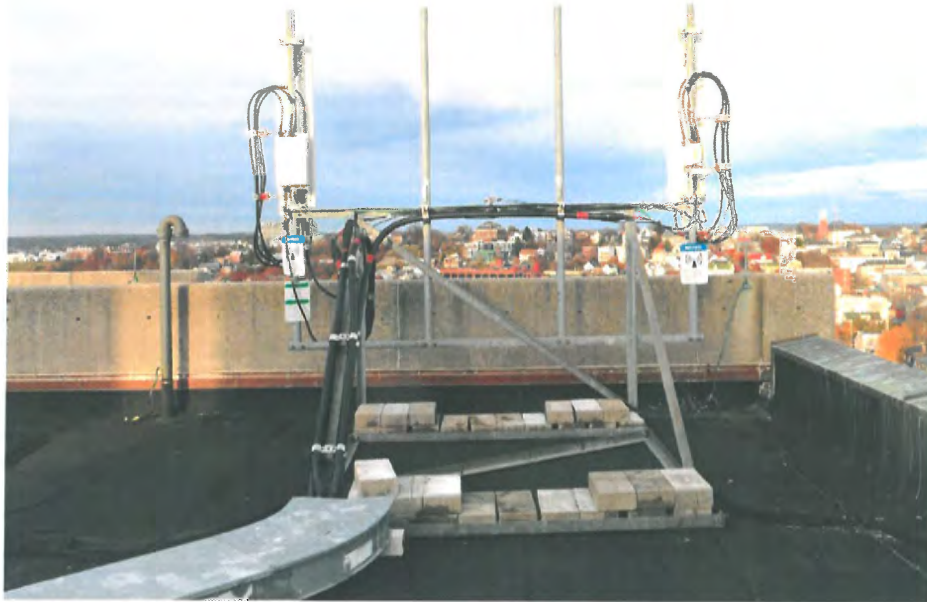
Photo 1: Sample photo illustrating the existing Alpha sector antennas.
