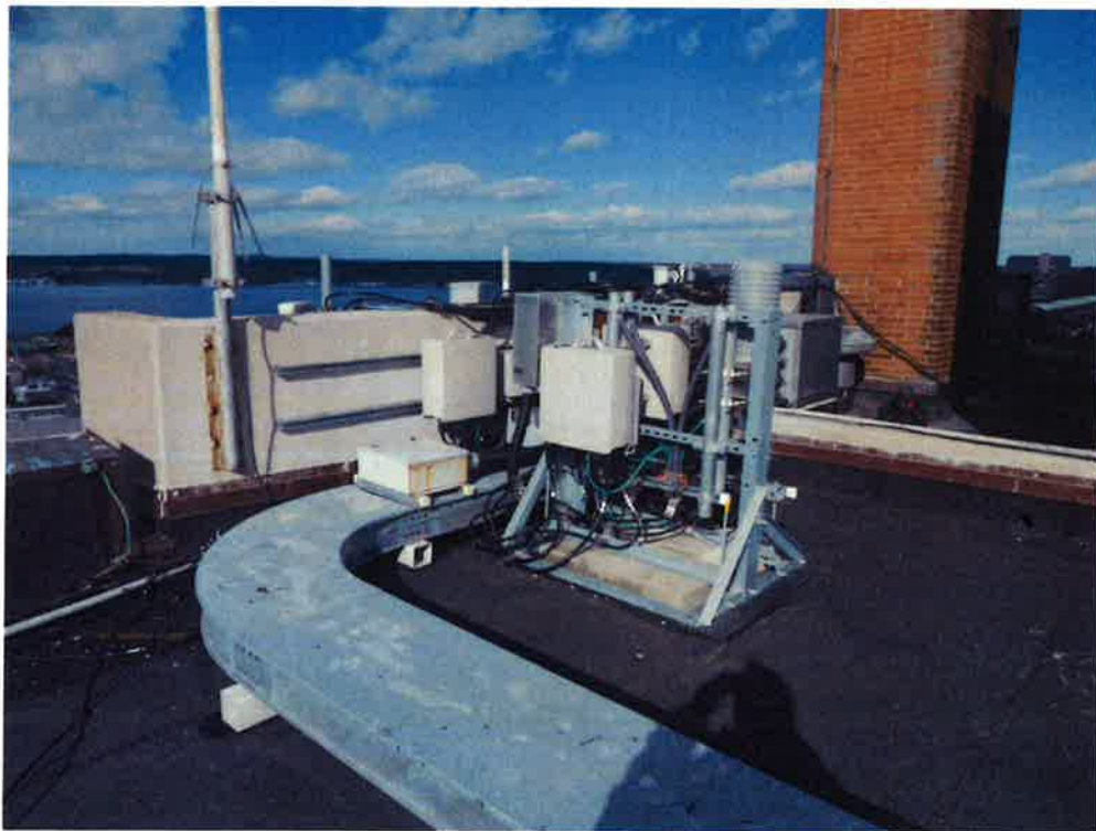
Photo 4: Sample photo illustrating the existing Gamma sector RRH's.
