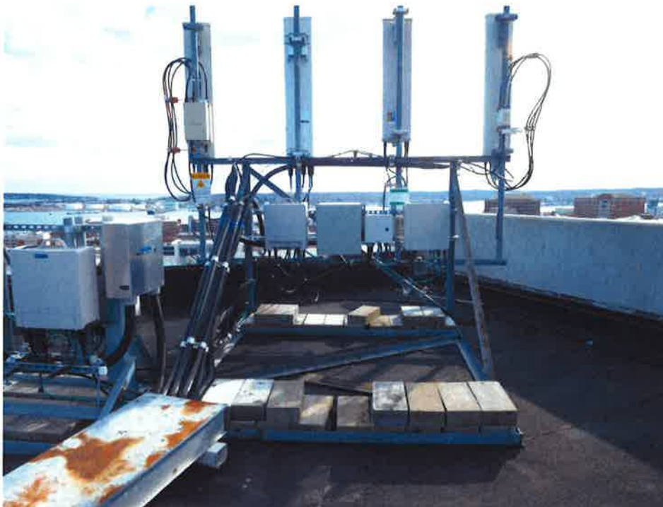
Photo 2: Sample photo illustrating the existing Beta sector antennas.
