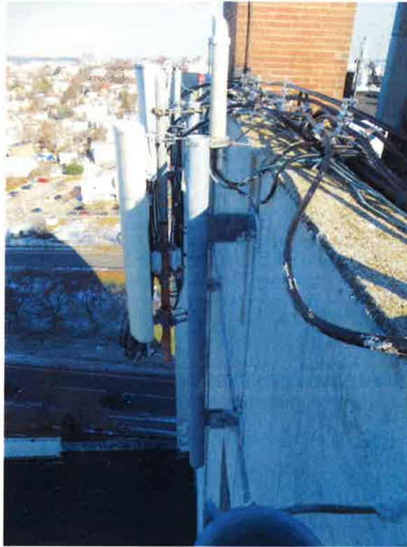
Photo 3: Sample photo illustrating the existing Gamma sector antennas.
