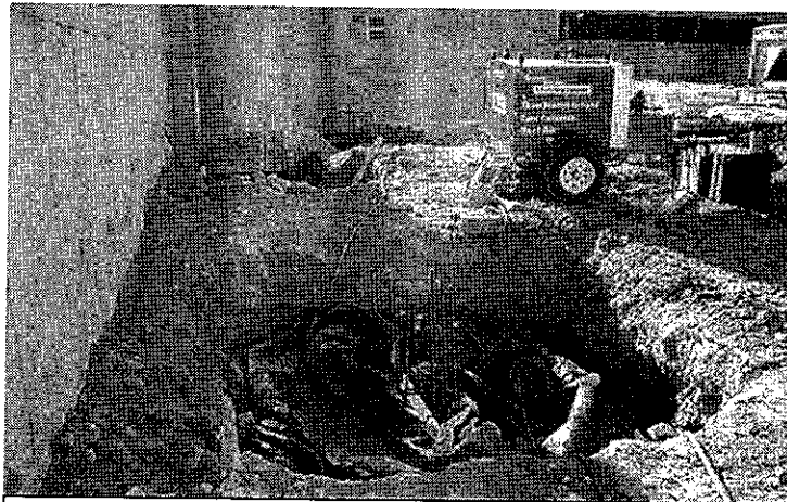
Photo 2: ground heater tendons draped inside forms for spread footing and covered with thermal blankets
