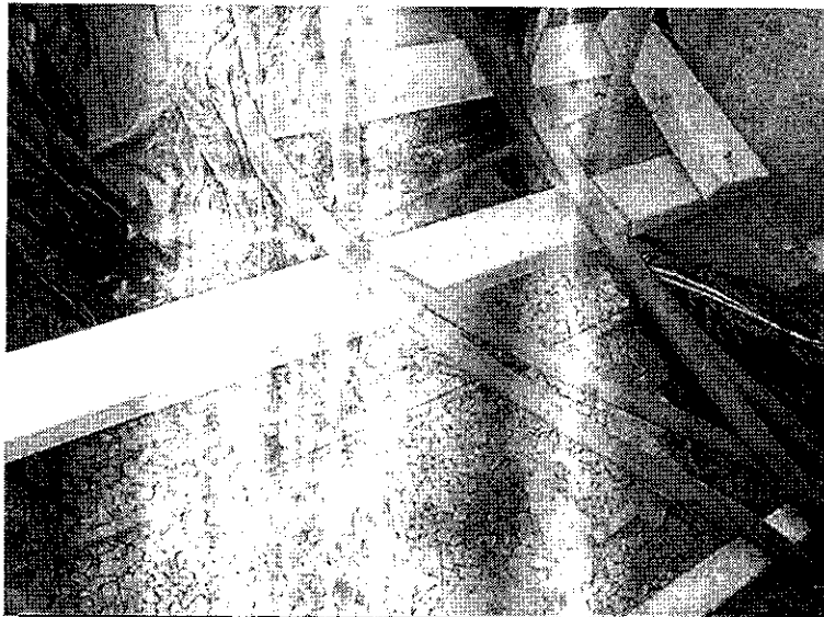
Photo 2: Ice within the formwork of today's proposed concrete placement
