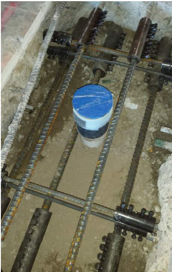
Photo 1: Cut Top/Bottom Bars Can't be coupled
