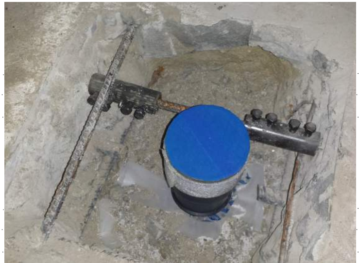
Photo 4: Cut Bottom Bar Cannot Be Lapped w/ New Couplers
