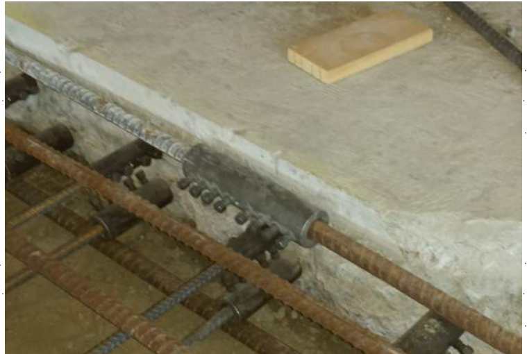
Photo 2: Coupler w/ Inadequate Cover
