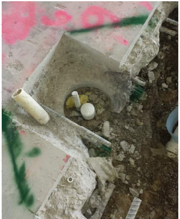
Photo 5: Existing slab cuts create re-entrant corners (green spray paint shows correct areas to be removed in the future)
