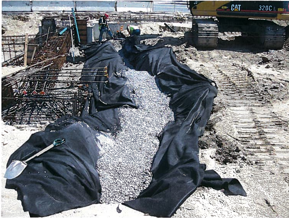
Photograph 3. Installation of the underslab drain running west to east between column lines G and H, looking east (7/25/07).
