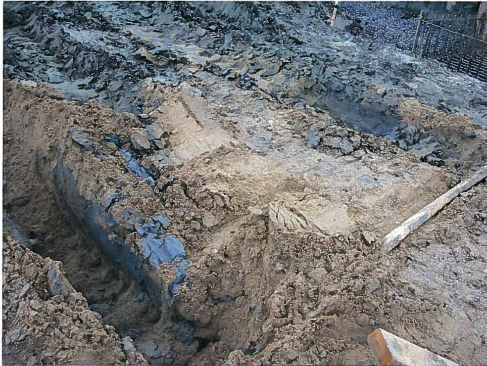
Photograph 1. Disturbed marine clay subgrade east of pile cap located at column line B-1. Disturbance caused by construction vehicle traffic, looking west (7/24/07).
