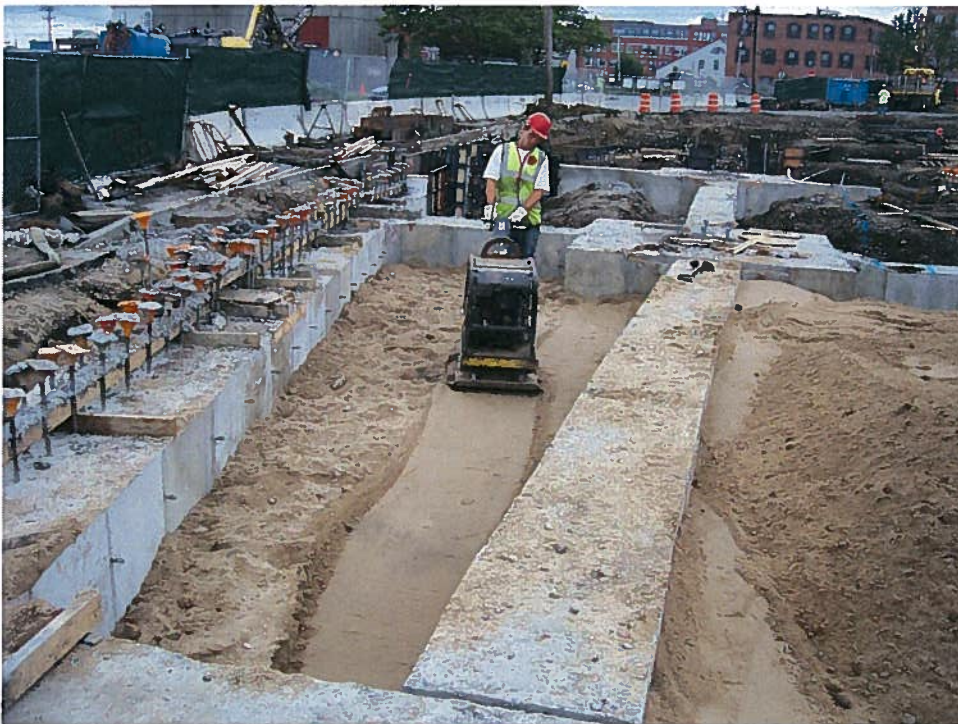
Photograph 2. Compacting granular backfill against pile caps/grade beams with a self-propelled vibratory plate compactor, looking south (7/24/07).
