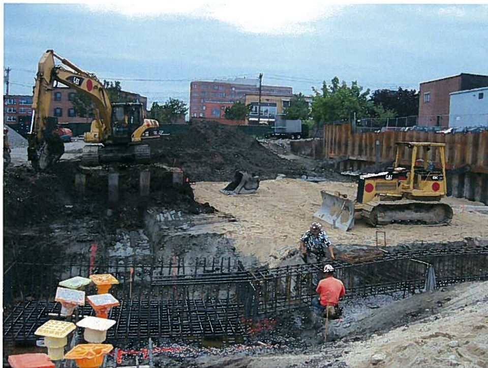
Photograph 2. Excavation of pile cap located at column line C-1.9/2.1 with granular fill subgrade protective layer visible to the right, looking south (7/18/07).
