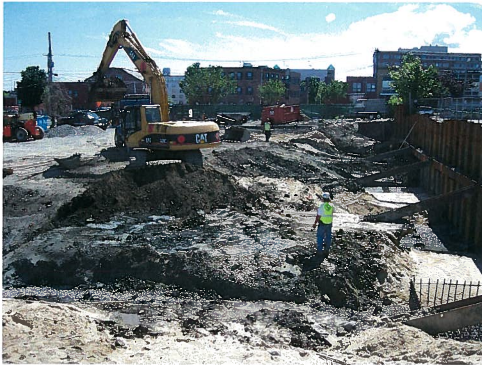
Photograph 1. Excavation to subgrade level south of column line D with exposed marine clay subgrade, looking south (7/19/07).
