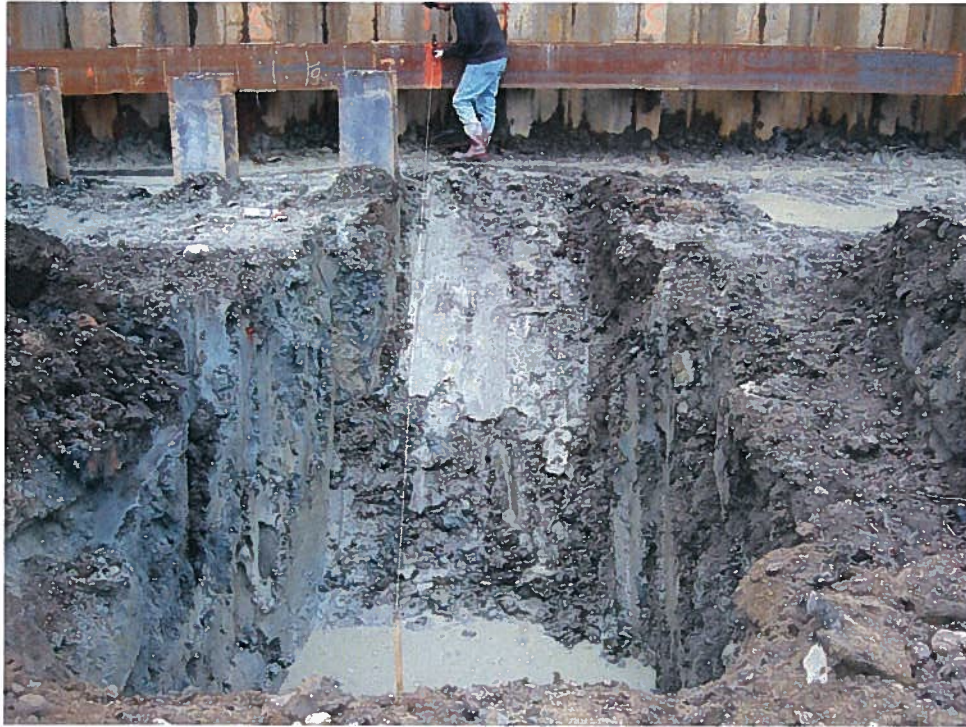
Photograph 1. Excavation of raker blocks for the support of excavation system along column line 1, looking west (7/9/07).
