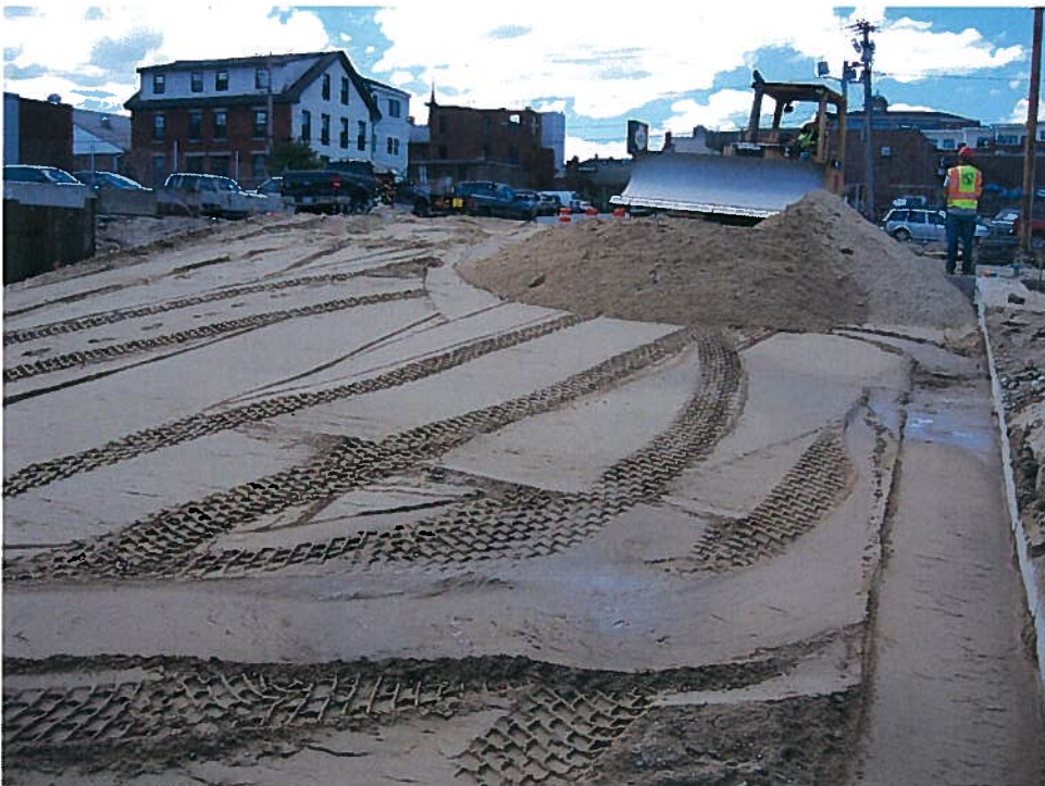
Photograph 6. Spreading a lift of granular fill in the northwest building corner with a CAT D5C bulldozer, looking west (7/13/07).
