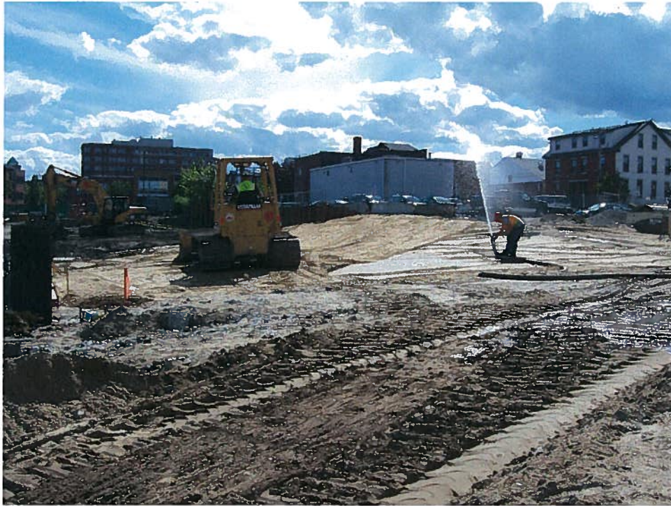
Photograph 5. Spreading a lift of granular fill in the northwest building corner and adding water for compaction, looking south (7/12/07)..
