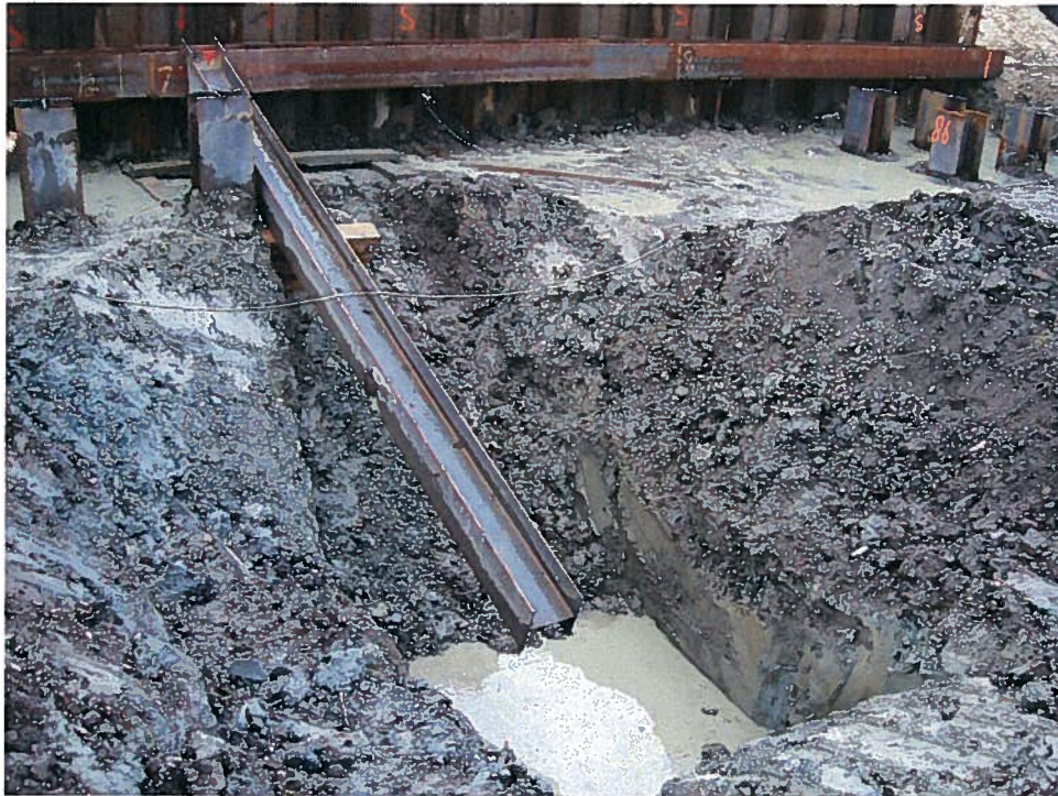
Photograph 2. Installation of rakers for the support of excavation system along column line 1, looking west (7/10/07).
