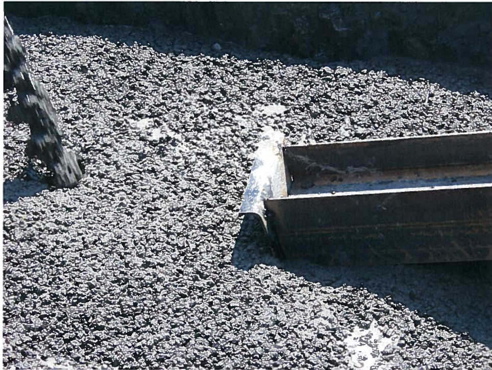
Photograph 3. Pouring concrete for raker blocks east of column line 1 with bearing plate visible on the end of the raker, looking south (7/10/07).
