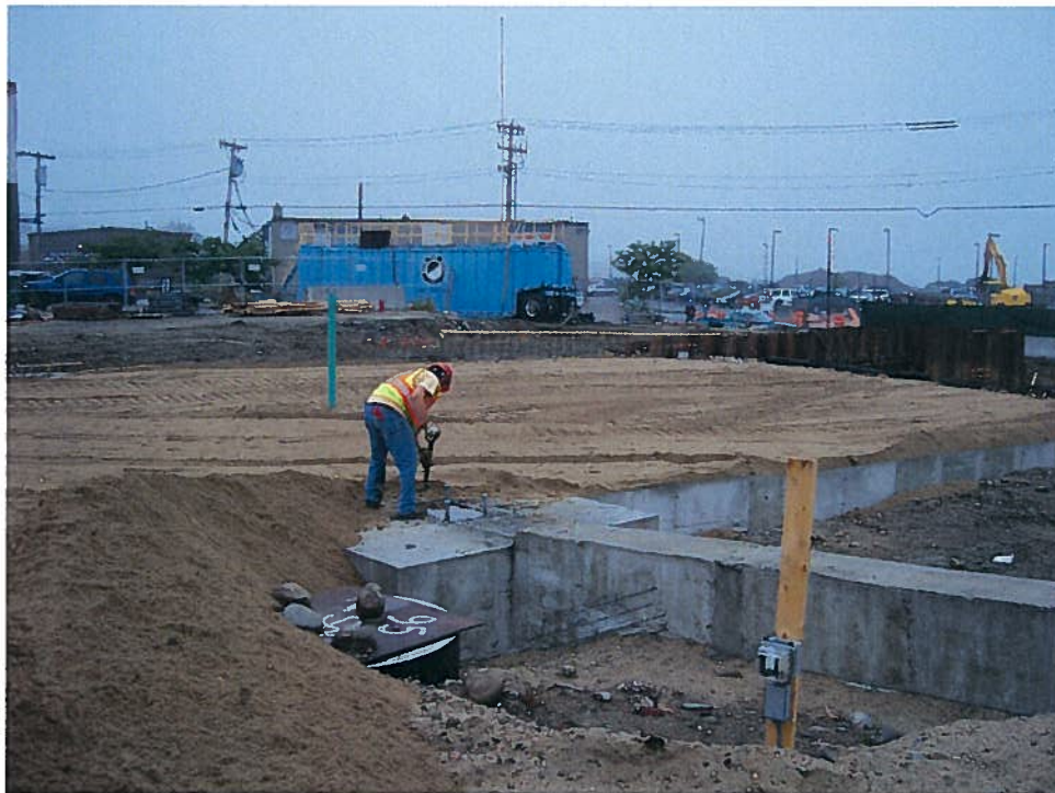
Photograph 4. Spreading lifts of granular fill in the northwest building corner, looking east (7/10/07).
