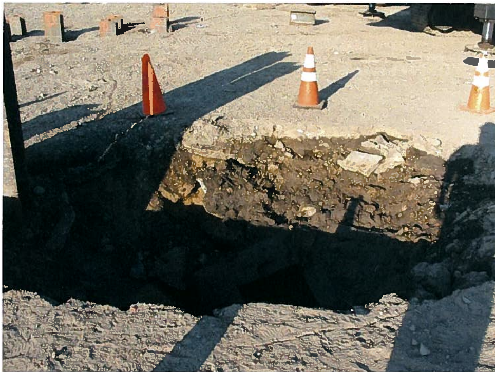
Photograph 2 Suspected underground storage tank near pile cap E-1.9/2.1 (6/18/07).
