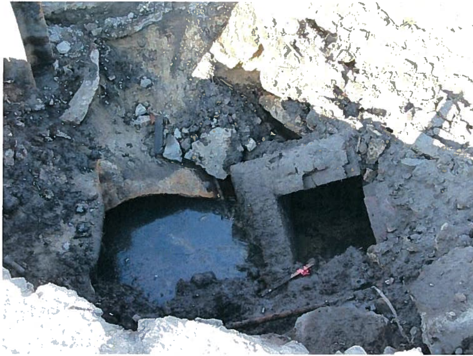
Photograph 1. Suspected underground storage tank near pile cap E-1.9/2.1 (6/18/07).
