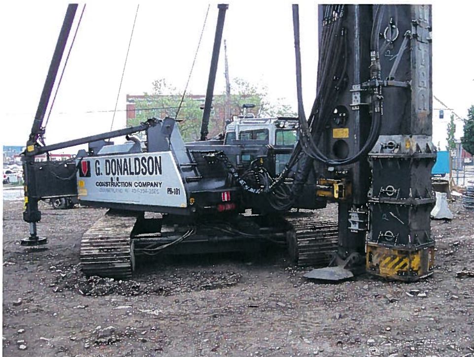
Photograph 6. The Junttan PM30 piling rig outfitted with a Junttan HHK-9A hydraulic hammer used to install indicator and production piles.
