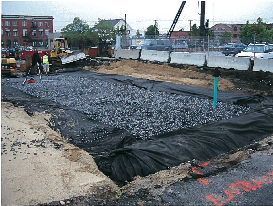
Photograph 4. Subsurface stormwater detention structure backfilled with 1½-in. crushed stone and partially wrapped with geosynthetic fabric, looking southeast (6/5/07).
