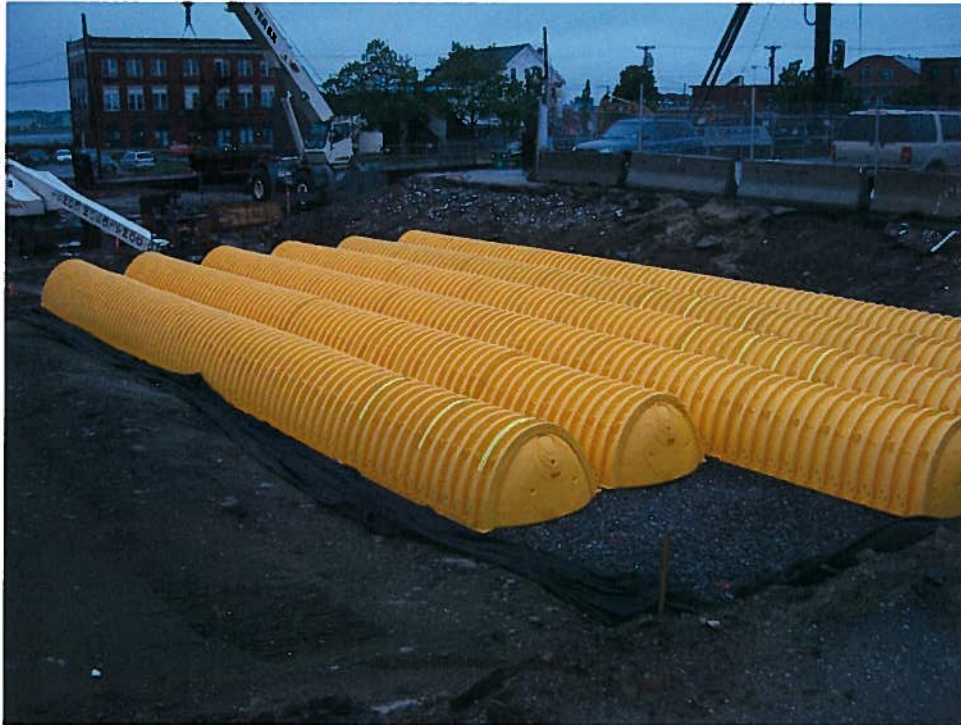
Photograph 1. Installed subsurface stormwater detention structure beneath the entrance roadway off of Middle Street, west of column line 1, looking east (6/4/07).
