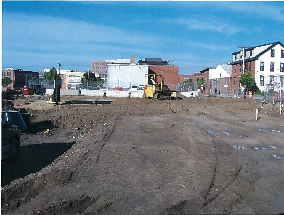
Photograph 5. Spreading a lift of aggregate subbase over the top of the subsurface stormwater detention structure and within the limits of the entrance roadway off of Middle Street, looking south (6/6/07).
