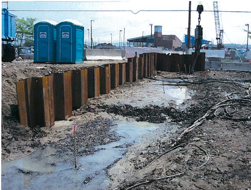
Photograph 3. Installing steel sheeting for the support of excavation system in the northeast building corner, along column line H, looking east (6/5/07).
