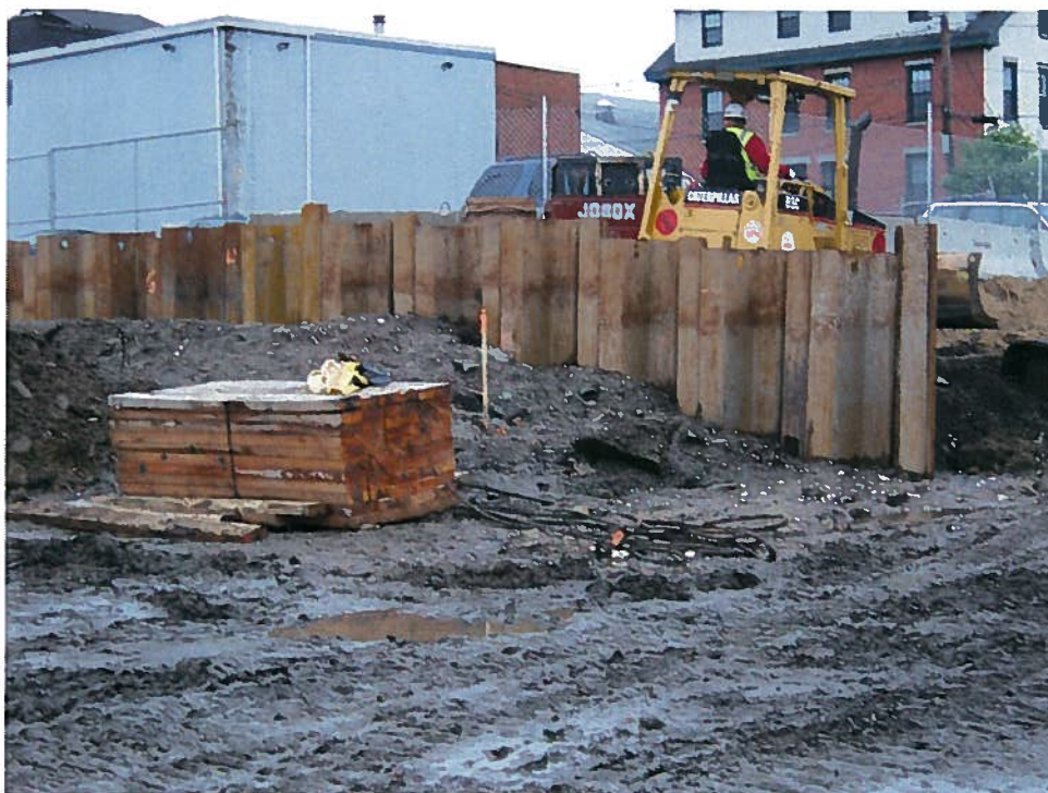
Photograph 2. End of sheeting installed for the support of excavation system parallel to column line 1 north of column line D, looking west (6/4/07).
