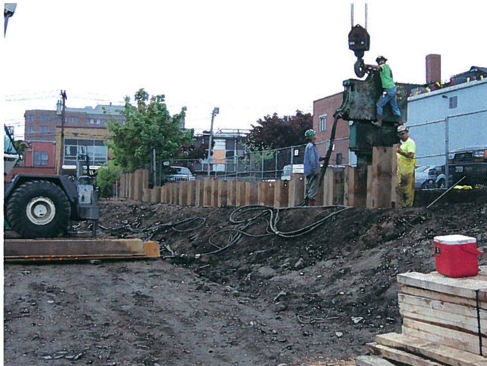
Photograph 6. Installation of steel sheeting for the support of excavation system parallel to column line 1, adjacent to the Micucci property, looking south (5/31/07).
