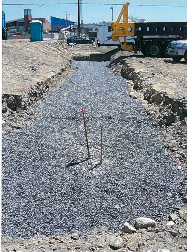
Photograph 1. Crushed stone placed over prepared subgrade along column line H, looking east (5/29/07).
