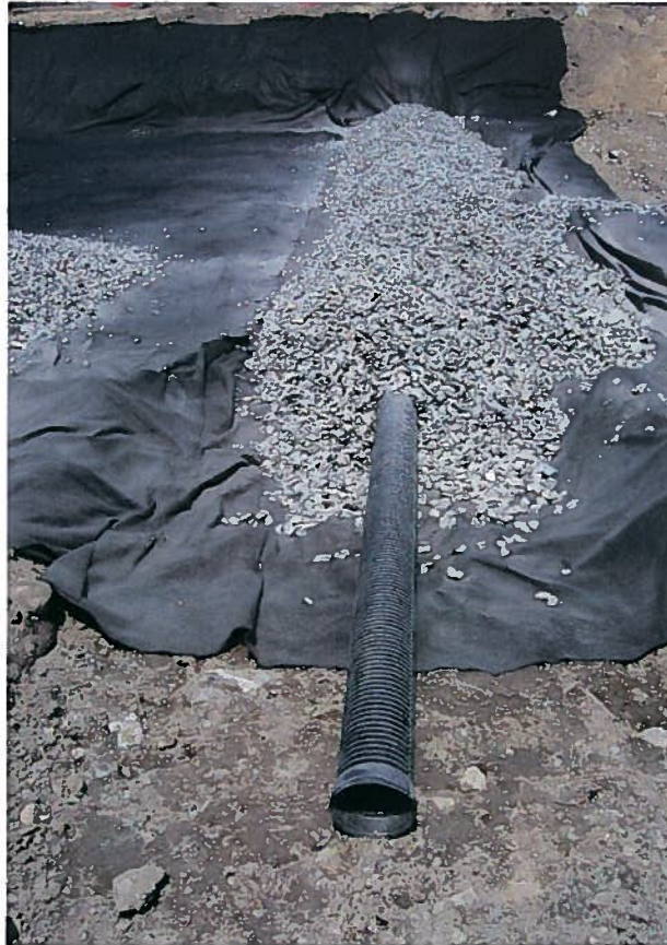
Photograph 4. 6-in. diameter perforated plastic underdrain pipe installed (invert at El. 19) beneath the subsurface stormwater chamber, looking west (5/30/07).
