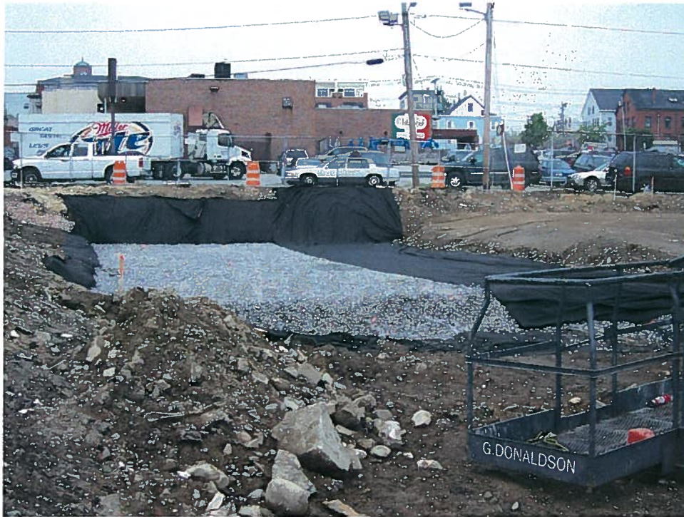
Photograph 5. Completed crushed stone layer (top at El. 20) beneath the proposed subsurface stormwater detention structure, looking west (5/30/07).
