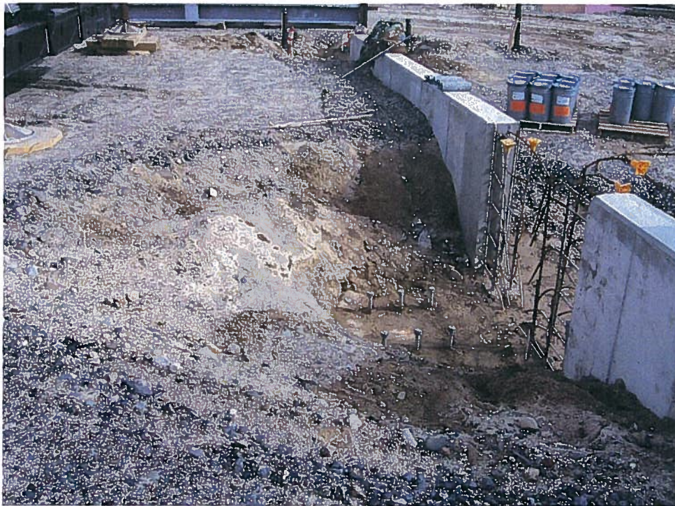
Photograph 2. Area at column line F-1.9/2.1 requiring backfilling and placement of subbase and base gravel after placement of steel superstructure and pouring the remaining portion of the wall, looking northeast (10/15/07).
