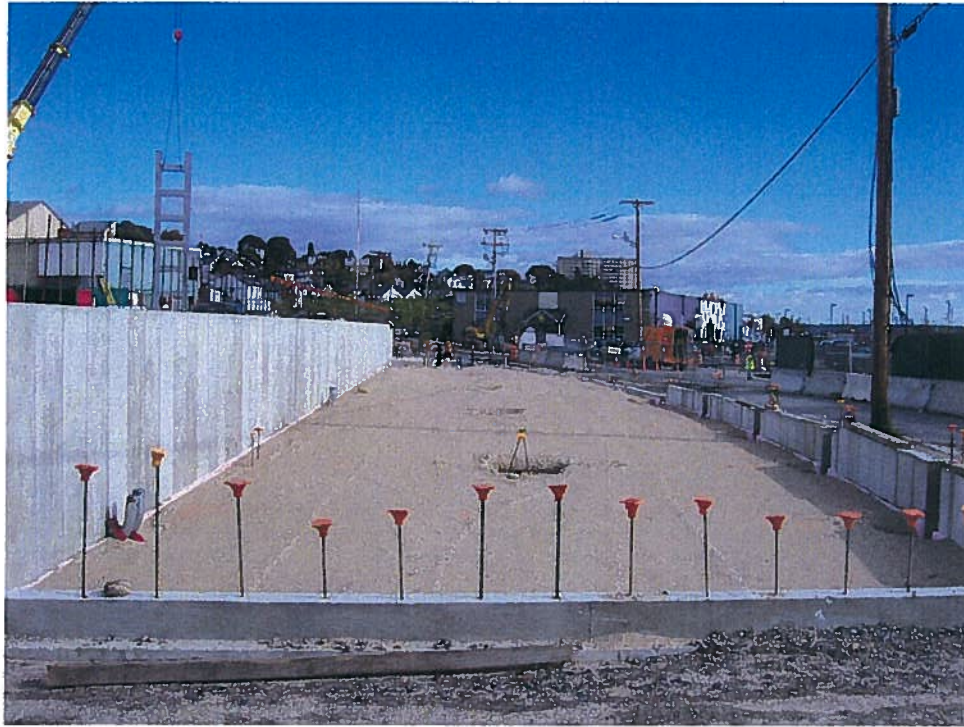
Photograph 3. Retail area space with imported granular fill placed/compacted up to the bottom of floor slab elevation (approximate), looking north (10/15/07).
