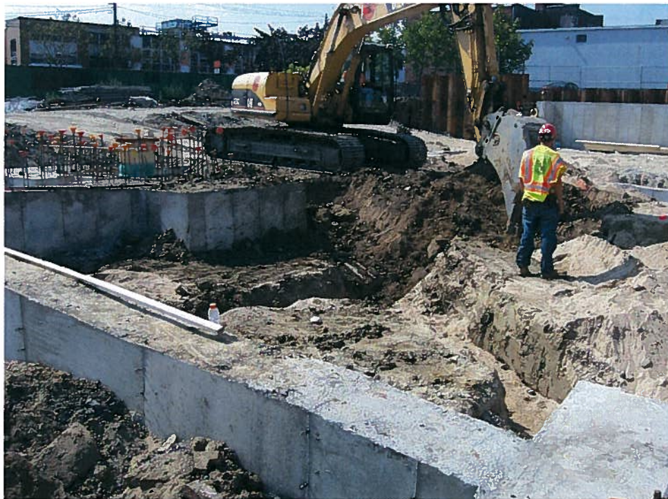
Photograph 6. Excavation for the oil/water separator in the southeast building corner, looking southwest (8/30/07).
