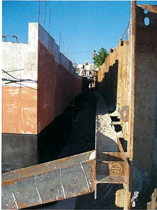
Photograph 1. Dampproofing and drainage board installed on the exterior side of the foundation wall along column line 1, from column line A to column line D, looking south (8/27/07).
