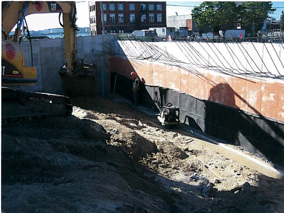
Photograph 2. Dampproofing and drainage board installed on the interior side of the foundation wall along column line D from column line 1 to column line 1.9/2.1, looking southeast (8/27/07).
