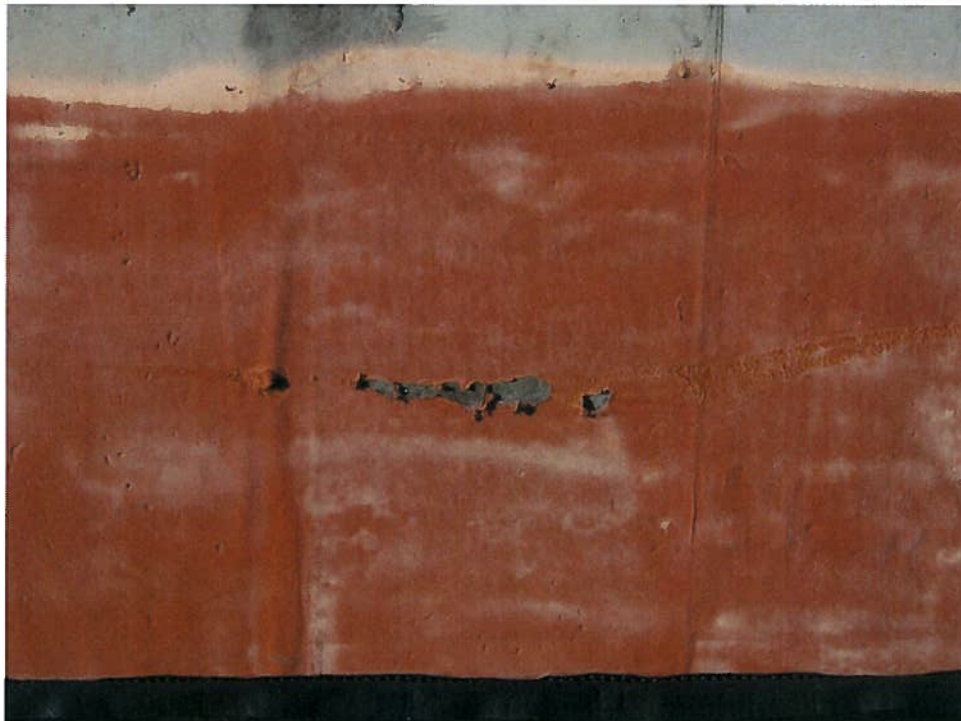
Photograph 4. Damaged waterproofing along column line D, looking south (7/28/07).
