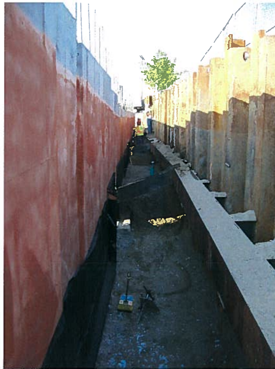
Photograph 5. Backfilling along column line 1 between the foundation wall and the steel sheet pile support of excavation system, looking south (8/30/07).
