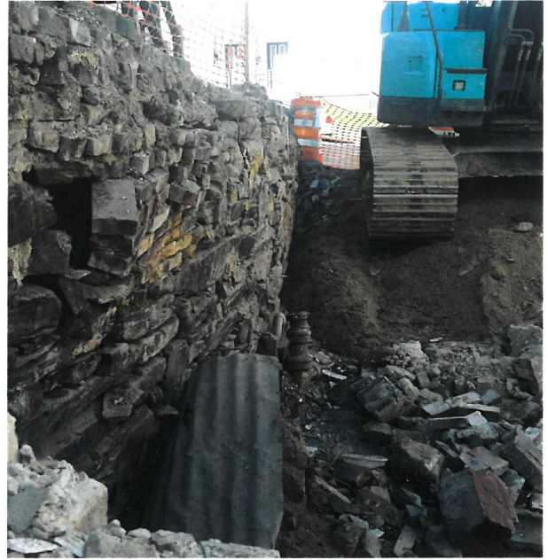
Picture 2: Deflection of Stone Foundation Wall
