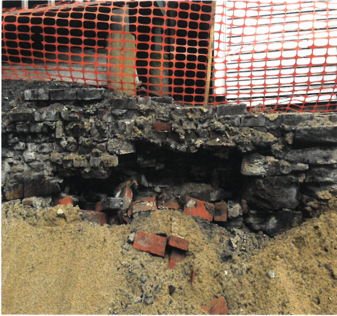
Picture 1: Crumbling Stone Foundation Wall
