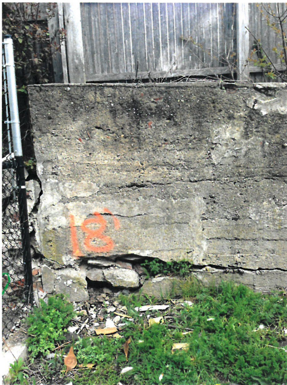
Picture 3: Large Void in Retaining Wall
