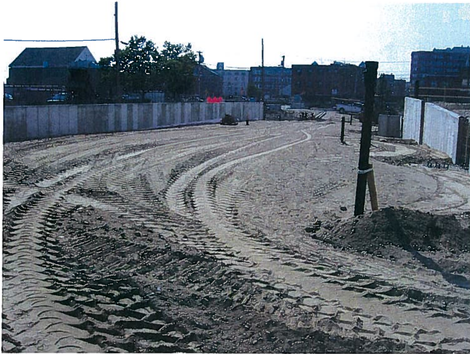
Photograph 1. Type D subbase gravel previously placed between column line 1.9/2.1 and 2.8, looking south (9/26/07).
