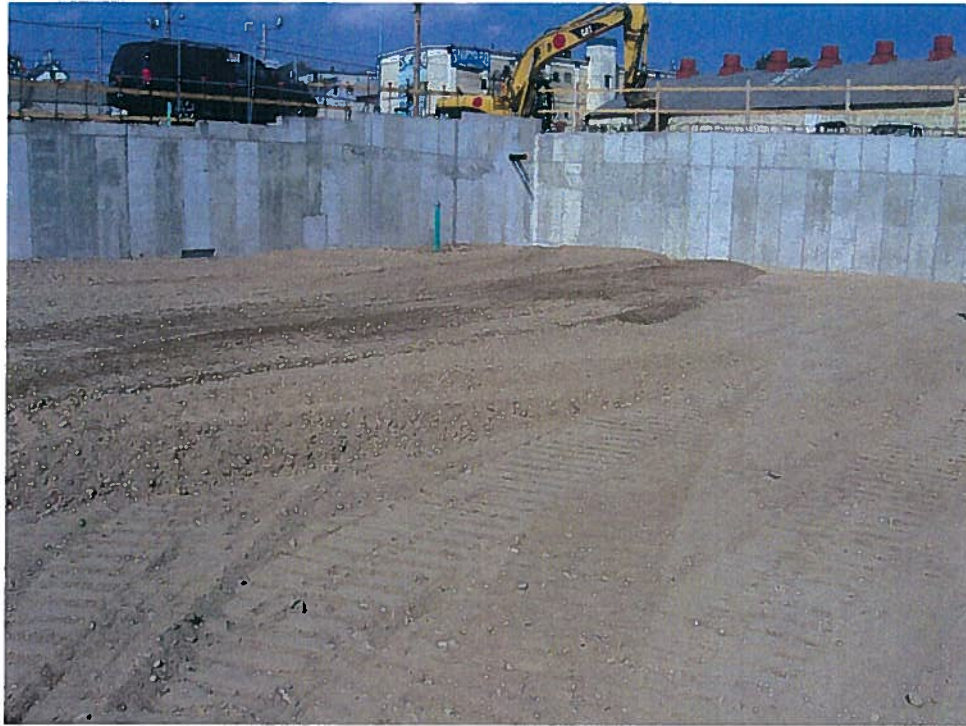
Photograph 3. Spreading a lift of Type A base gravel in the area between column lines 1, 1.9/2.1, D and C, looking northwest (9/26/07).
