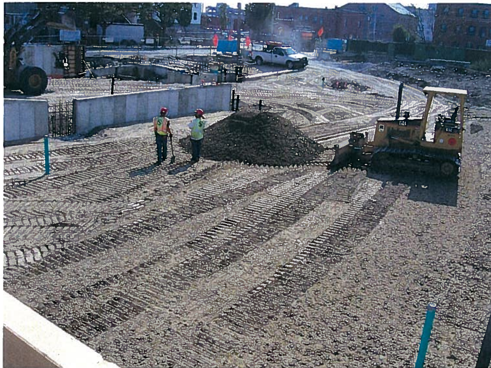
Photograph 4. Spreading a lift of Type A base gravel in the area between column lines 1, 1.9/2.1, D and C with a CAT D5C bulldozer, looking southeast (9/26/07).
