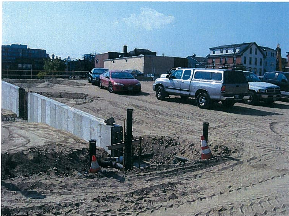
Photograph 2. Type D subbase gravel previously placed between column lines 1, 1.9/2.1, D and G, looking southwest (9/26/07).
