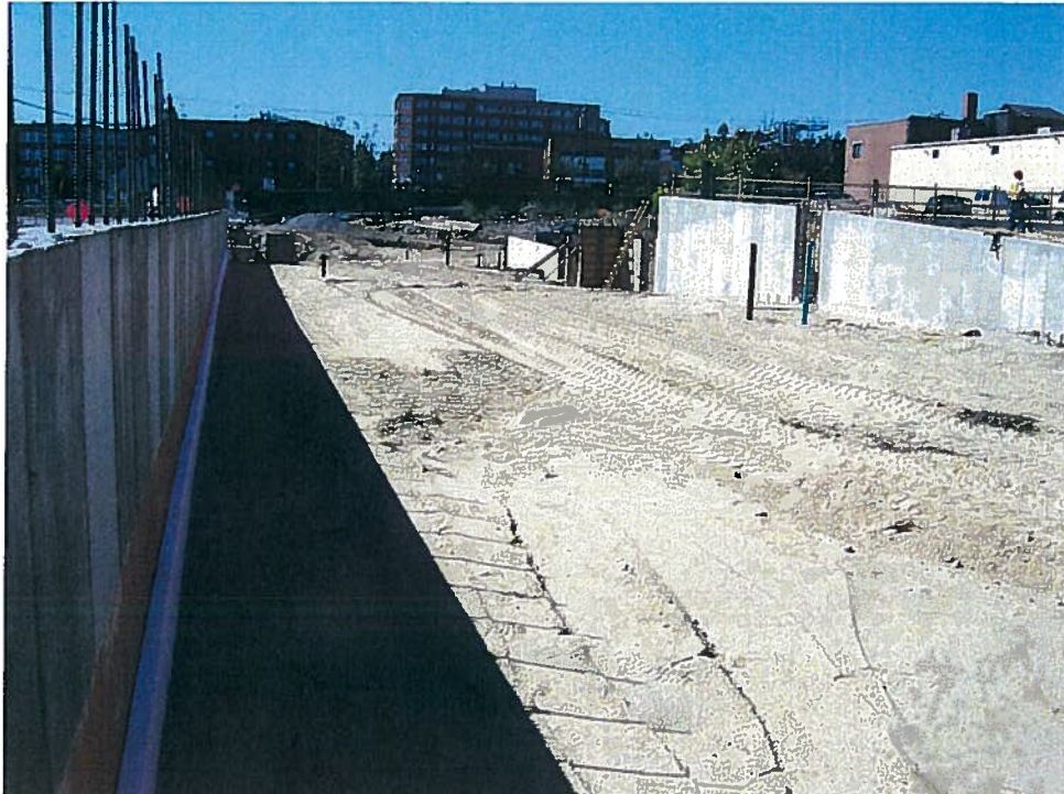
Photograph 1. Granular fill previously placed up to subgrade level between column line 1.9/2.1 and 2.8 with insulation board and waterproofing visible on the above grade wall along column line 2.8, looking south (9/17/07).
