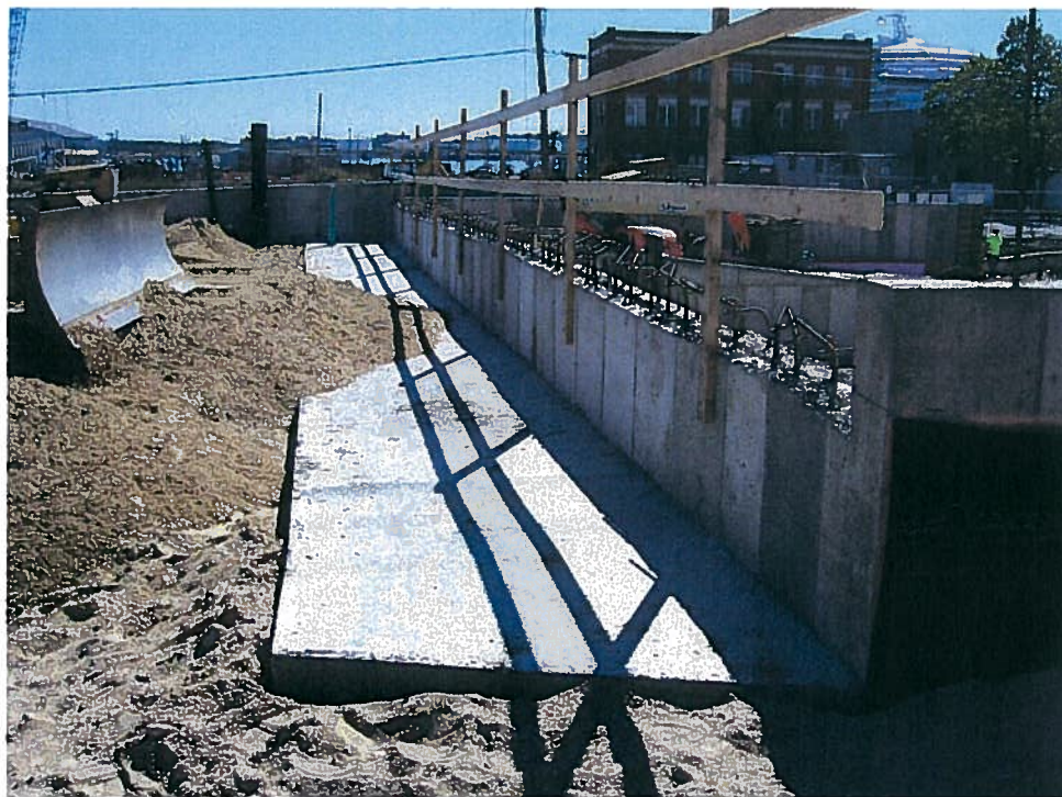
Photograph 4. Spreading a lift of granular fill up to subgrade elevation between column line 1 and column line 1.9/2.1 near column line D with a CAT D5C bulldozer, looking east (9/17/07).
