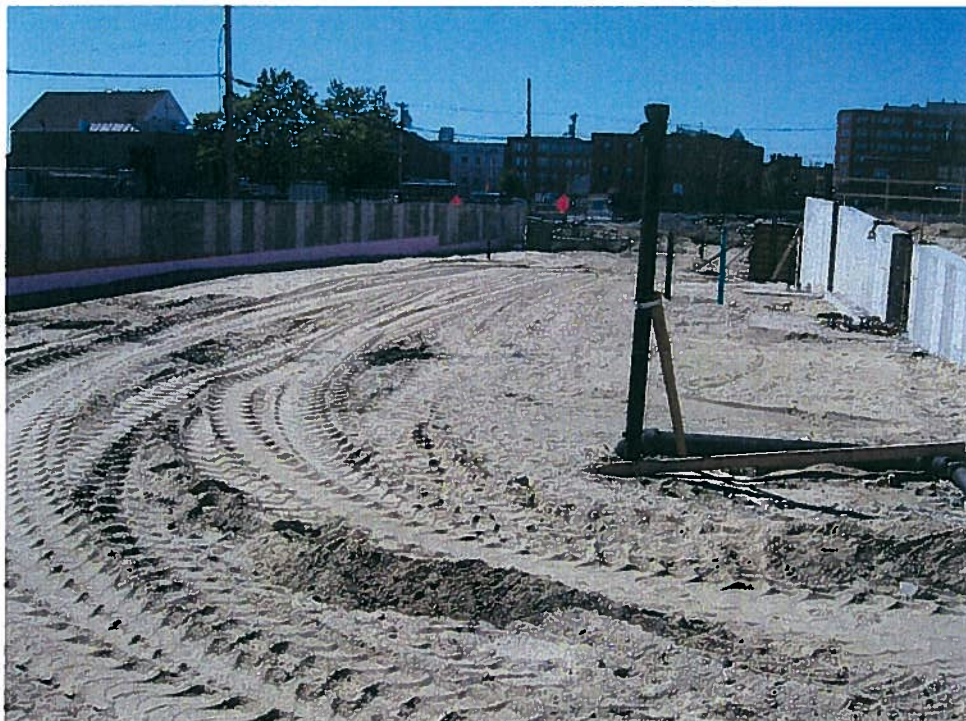
Photograph 2. Granular fill previously placed up to subgrade level between column line 1.9/2.1 and 2.8 with insulation board and waterproofing visible on the above grade wall along column line 2.8, looking south (9/17/07).
