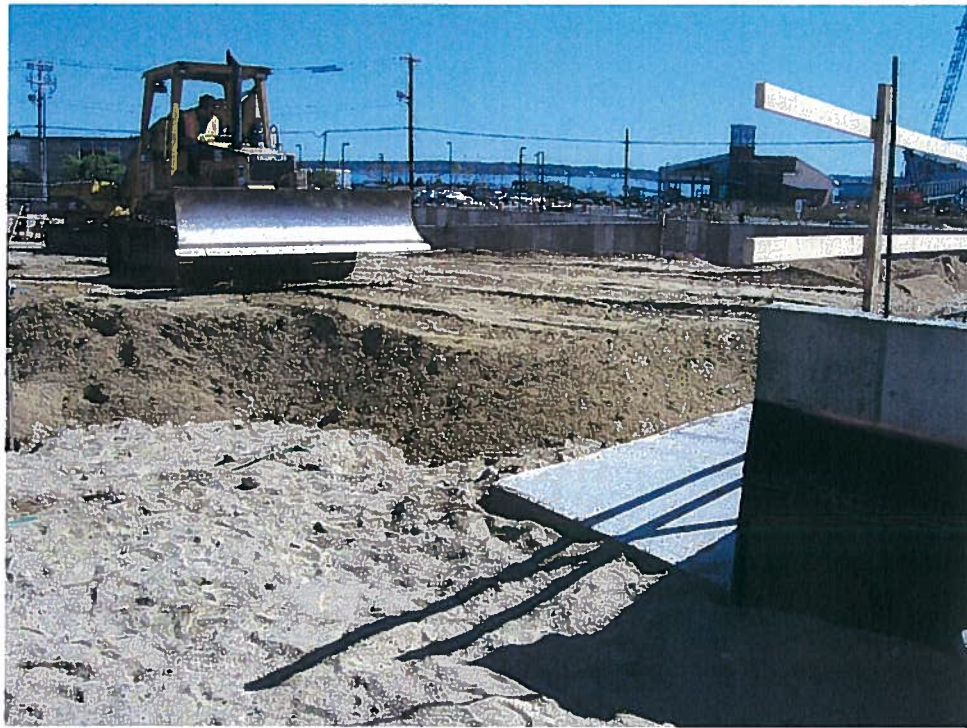
Photograph 3. Spreading a lift of granular fill up to subgrade elevation between column line 1 and column line 1.9/2.1 near column line D with a CAT D5C bulldozer, looking northeast (9/17/07).
