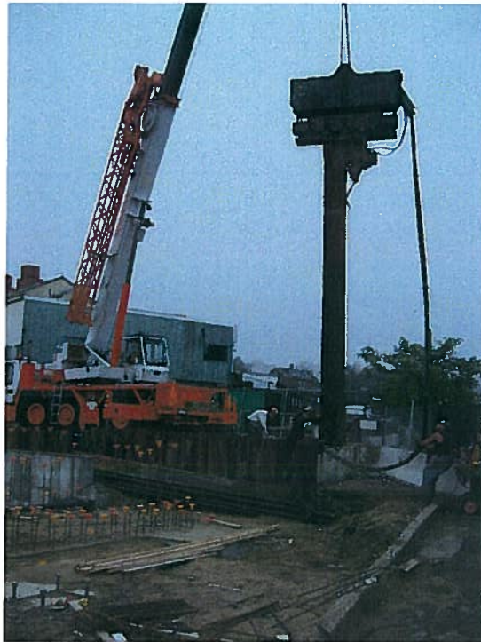
Photograph 3. Removal of steel sheet piles from the support of excavation system in the northeast corner of the garage, looking north (9/10/07).
