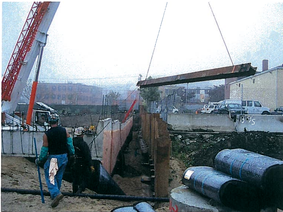
Photograph 2. Removal of the continuous steel waler for the support of excavation system west of column line 1, looking south (9/10/07).
