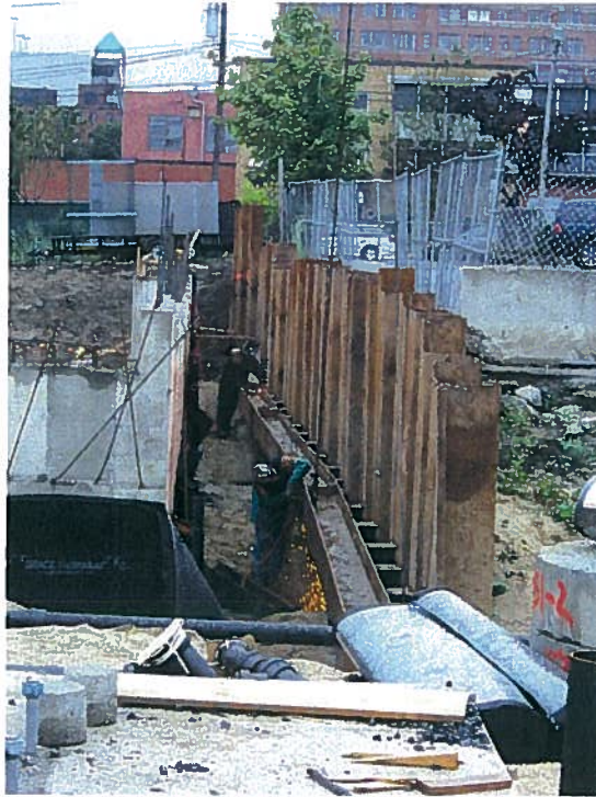
Photograph 1. Removal of the continuous steel waler for the support of excavation system west of column line 1, looking south (9/10/07).
