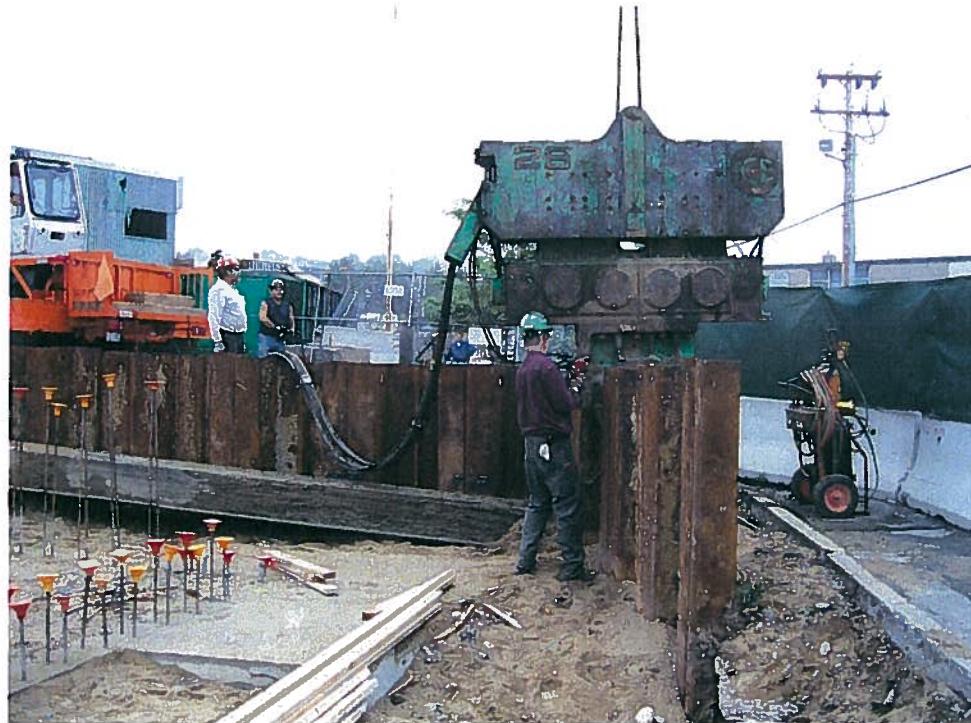
Photograph 4. Removal of steel sheet piles from the support of excavation system in the northeast corner of the garage, looking north (9/10/07).
