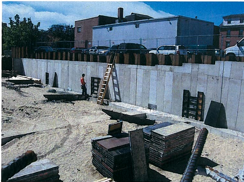
Photograph 2. Forming of cutouts in the foundation wall after removal of the rakers for the support of excavation system along column line 1, looking southwest (9/4/07).
