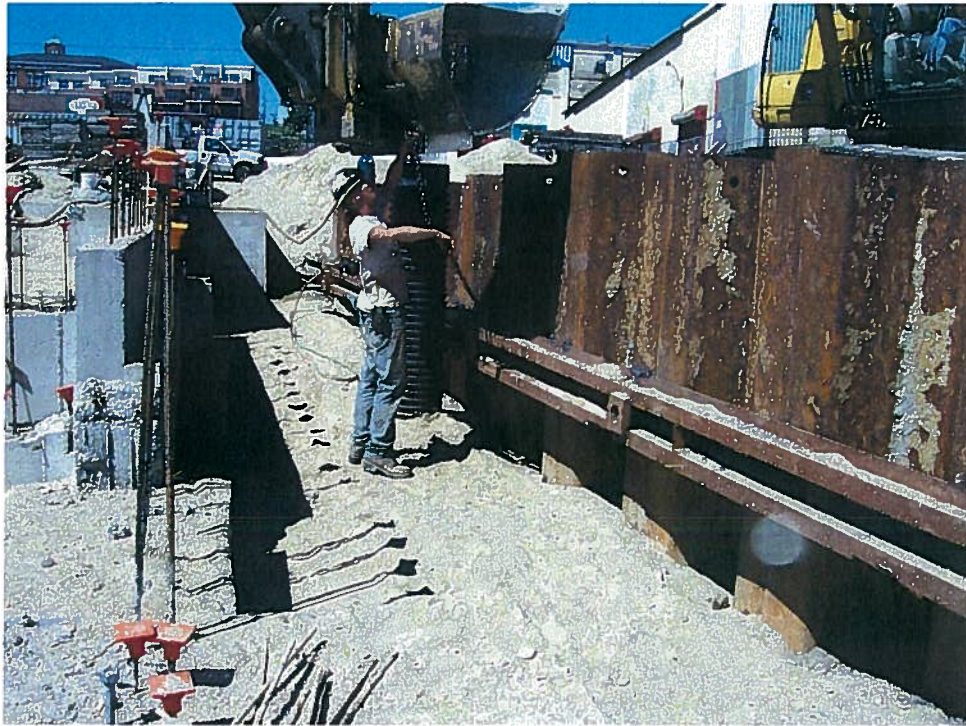
Photograph 3. Removal of the continuous steel waler from the support of excavation system north of the elevator pit in the northeast building corner, looking west (9/4/07).
