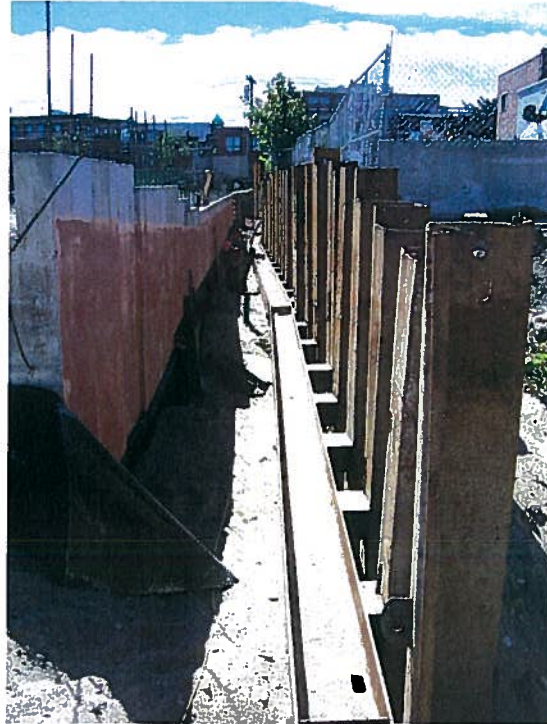
Photograph 1. Removal of rakers for the support of excavation system along column line 1, looking south (9/4/07).
