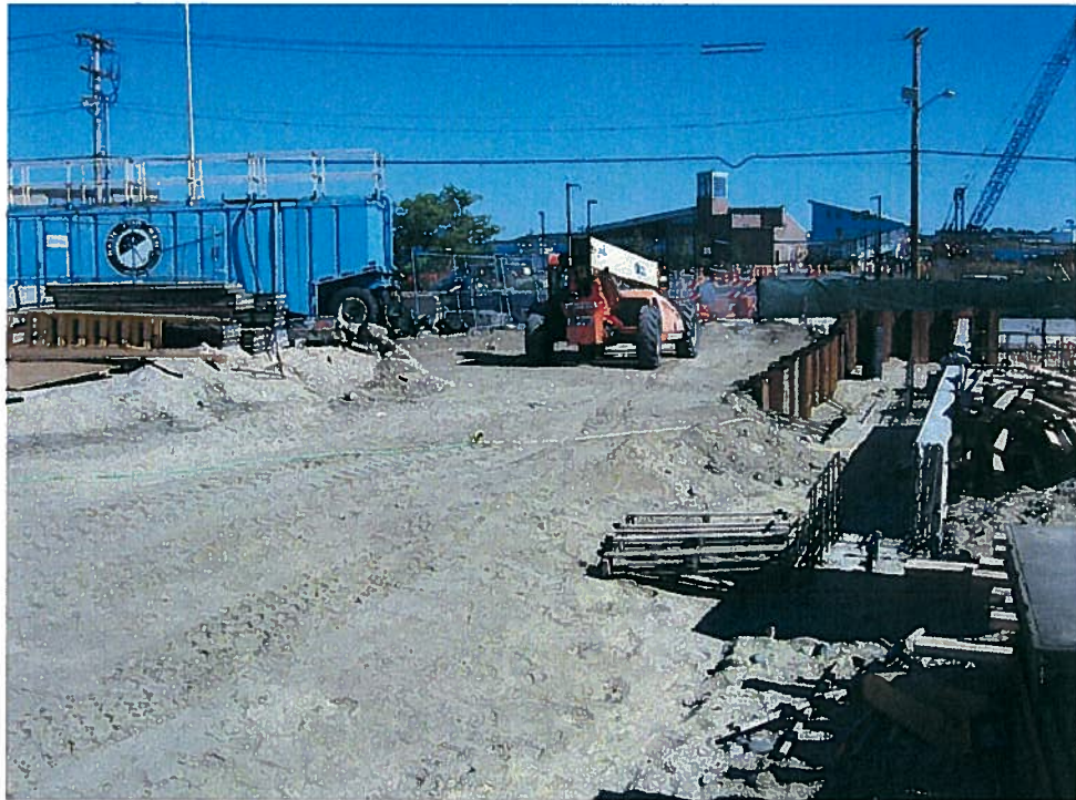
Photograph 4. Area north of the support of excavation system in the northeast building corner after removal of the concrete jersey barrier deadmen, looking east (9/5/07).
