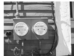
Existing Meter Panel
