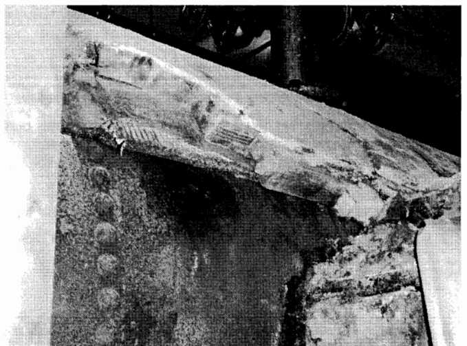
12 Emerson Street: Asbestos-containing boiler casing (ASB-105A) – Boiler 1
