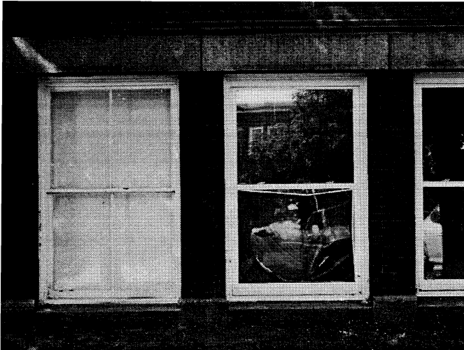
12 Emerson Street: Asbestos-containing exterior window glaze (ASB-121A) and window Caulk (ASB-122A)
