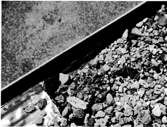
56 North Street: Asbestos-containing roof flashing (ASB-02A)
