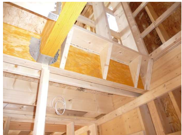
Photo #10 – 1 st Flr: Inadequate wall support
