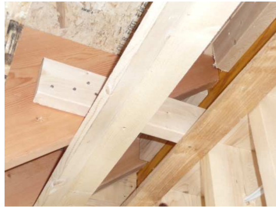
Photo #16 – 2 nd Flr: Center stringer needs ledger
