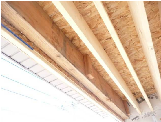
Photo # 15 – 2 nd Flr: Blocking needed @ guardrail post
