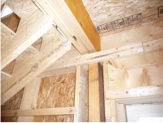
Photo # 13 – 1 st Flr: LVL 6’ Stringer sisters required
