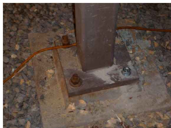
Photo #6 – Expansion bolt replaces missing anchor
