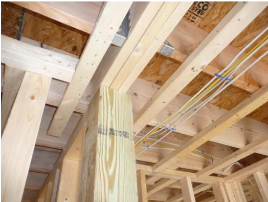
Photo # 21 – 3 rd Flr: Missing beam/column connector
