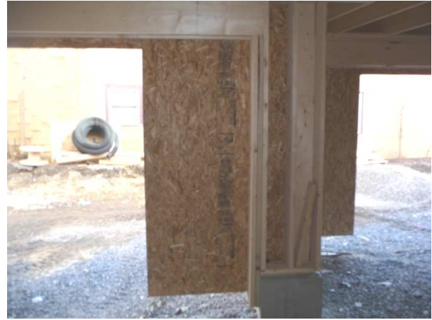
Photo #8 – Jack studs must be pressure treated
