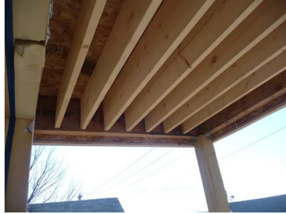
Photo #14 – 2 nd Flr: Porch hangers needed
