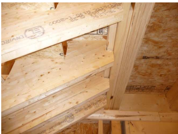
Photo # 11 – 1 st Flr: Inadequate stringer connection
