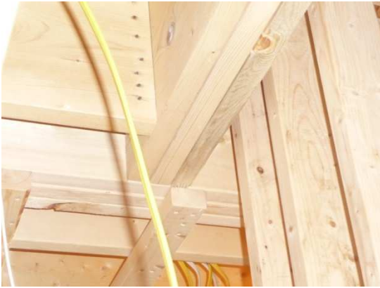
Photo # 29 – 2 nd Flr: Missing beam and joist hangers
