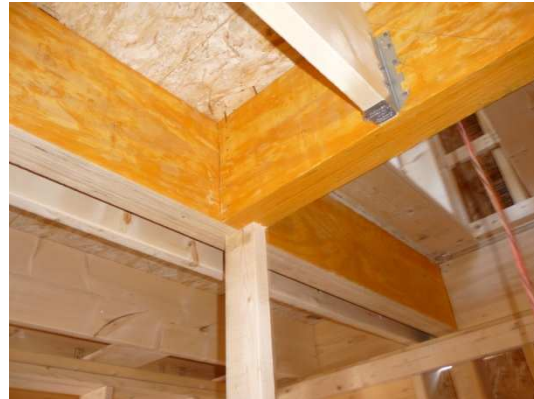
Photo #2 – Missing beam hanger
