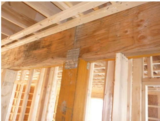
Photo # 3 – Nails missing at beam/column connectors
