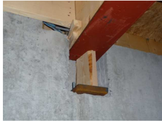
Photo #2 – Unacceptable steel beam support
