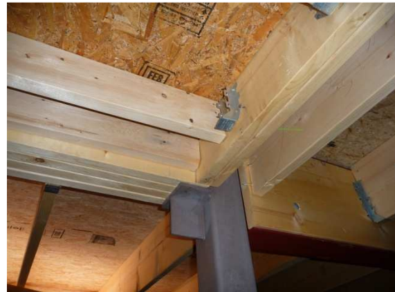
Photo #4 – Hangers missing at some joists
