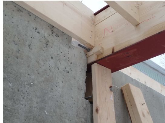
Photo #2 – Concrete beam pocket was too low
