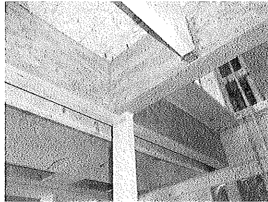
Photo #2 – Missing beam hanger
