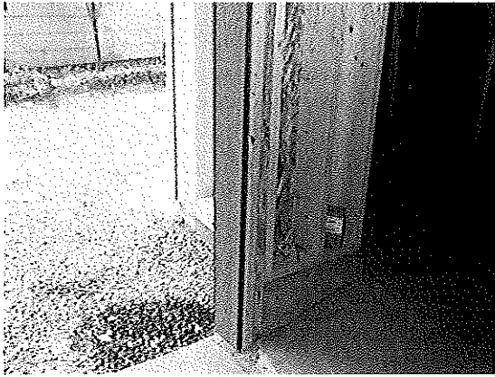
Photo #2 – Pressure treated jack studs at doors
