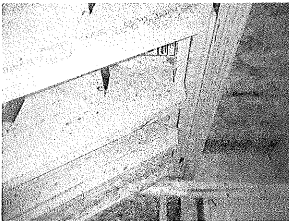
Photo # 11 – 1 st Flr: Inadequate stringer connection
