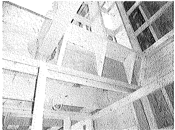
Photo #10 – 1 st Flr: Inadequate wall support
