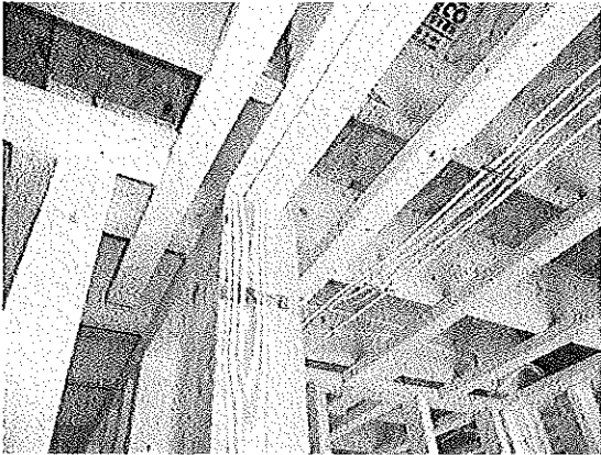
Photo # 21 – 3 rd Flr: Missing beam/column connector
