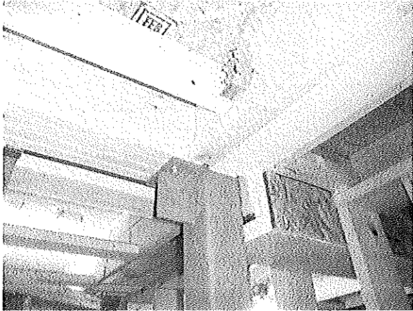
Photo # 7 –Joist needs hanger; double 2x beam needs post
