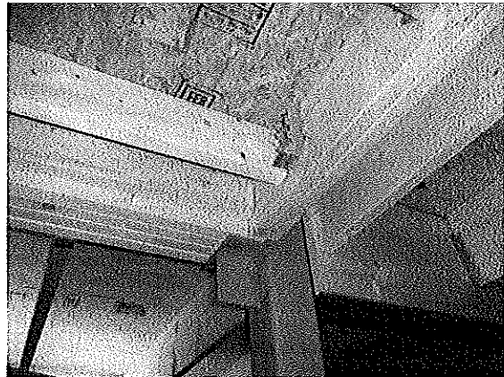
Photo #4 – Hangers missing at some joists
