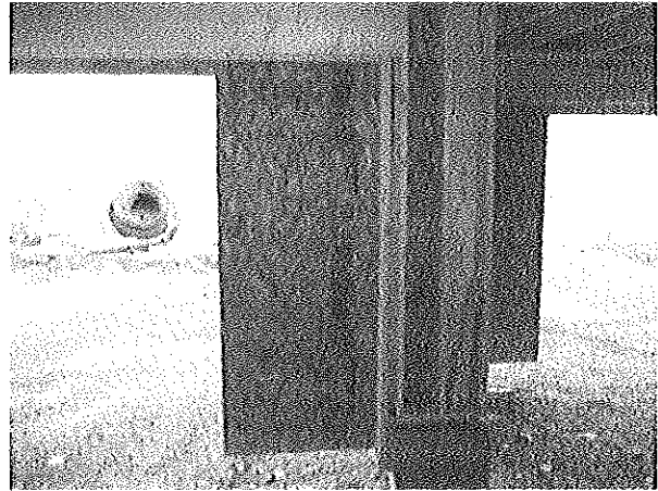
Photo #8 – Jack studs must be pressure treated
