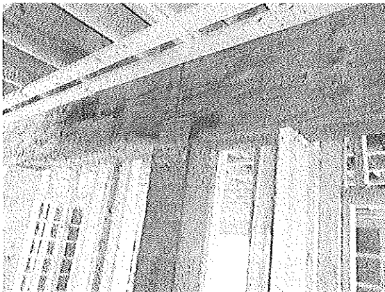
Photo # 3 – Nails missing at beam/column connectors
