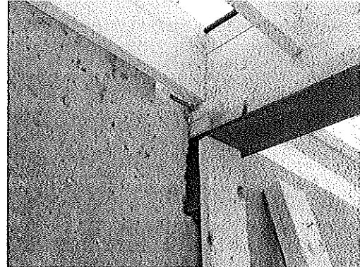
Photo #2 – Concrete beam pocket was too low
