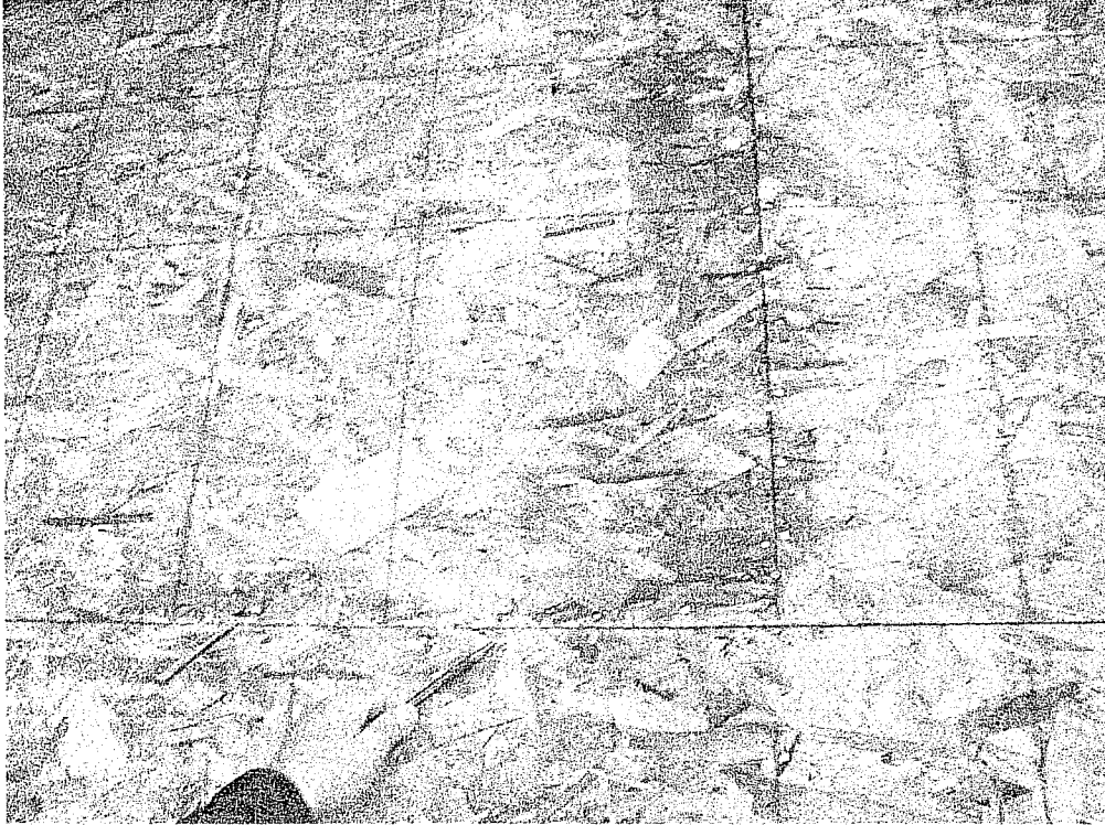
Photo 3 – Note the close spacing of nails at edges of always be sheathing. This was observed at shear wall construction.
