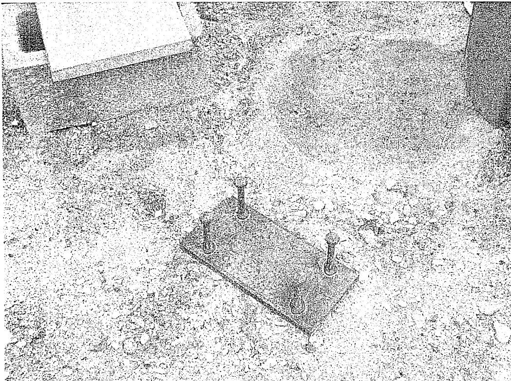
Photo 4 – Structural bearing plate with welded studs to be used at steel beams bearing on masonry.
