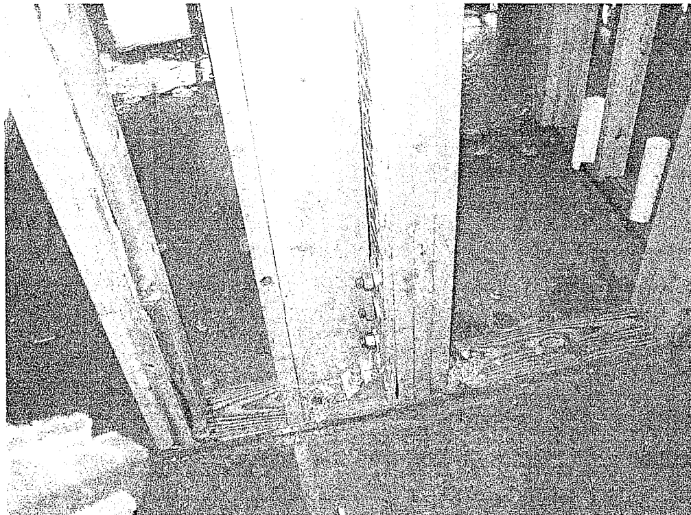
Photo 4 – Typical hold down anchor at top and bottom of shear walls
