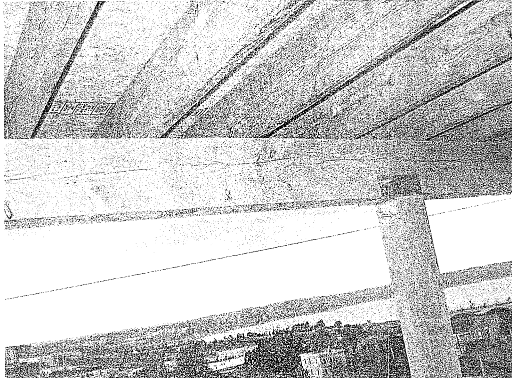
Photo # 4 - Note bolts at Column to Beam Connection. Also note Simpson connectors at Joists to Beam.
