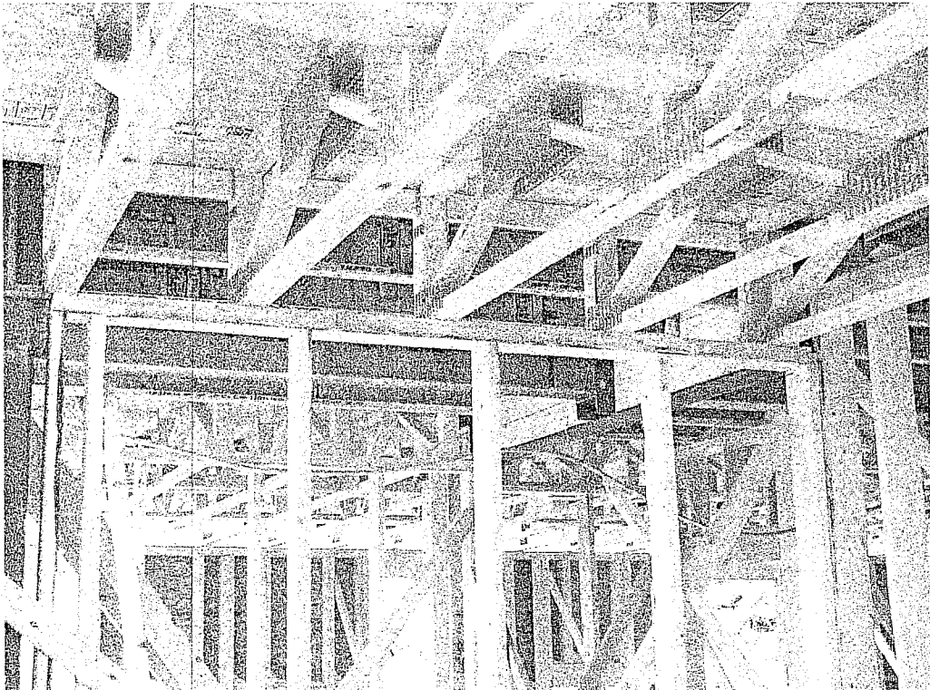
Photo 4 – Additional wall studs need to be added such that a stud aligns below centerline of each truss.
