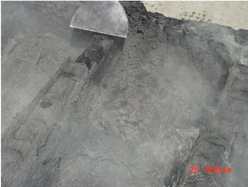
Photograph 11: Intumescent being scraped away to show char depth
