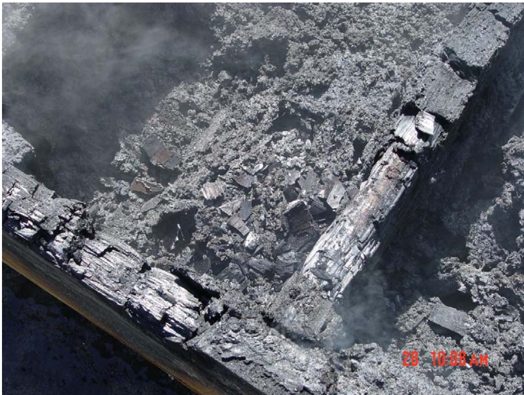
Photograph 12: Exposed sample with coating scraped away
