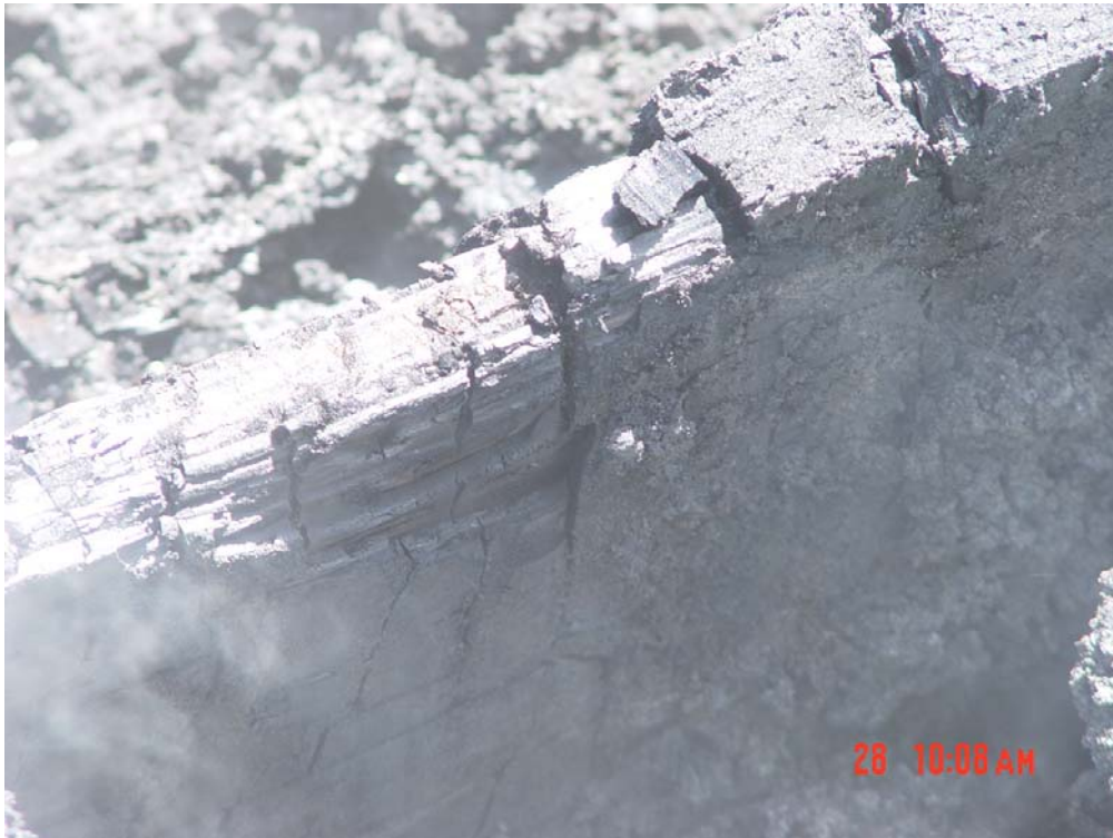
Photograph 13: Close-up of an exposed joist with the intumescent scraped off
