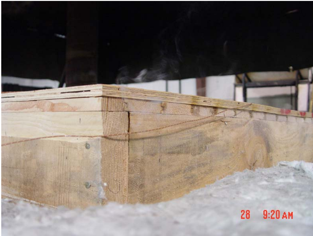
Photograph 5: Light smoke leaking through the tongue and groove layer
