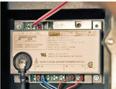
Fenwal ignition module - DC Microamp ( \mu A) test points are shown at top left corner of module (beside red L.E.D.)
