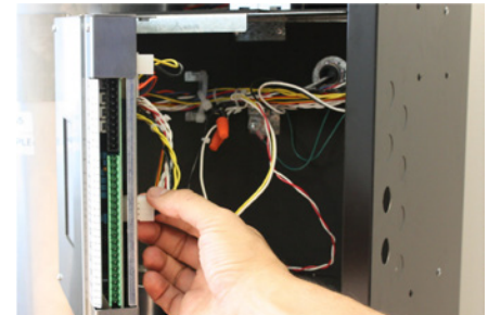
Control Module disconnection
