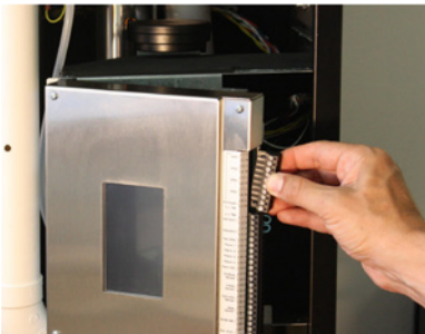
Line voltage load pump terminals
