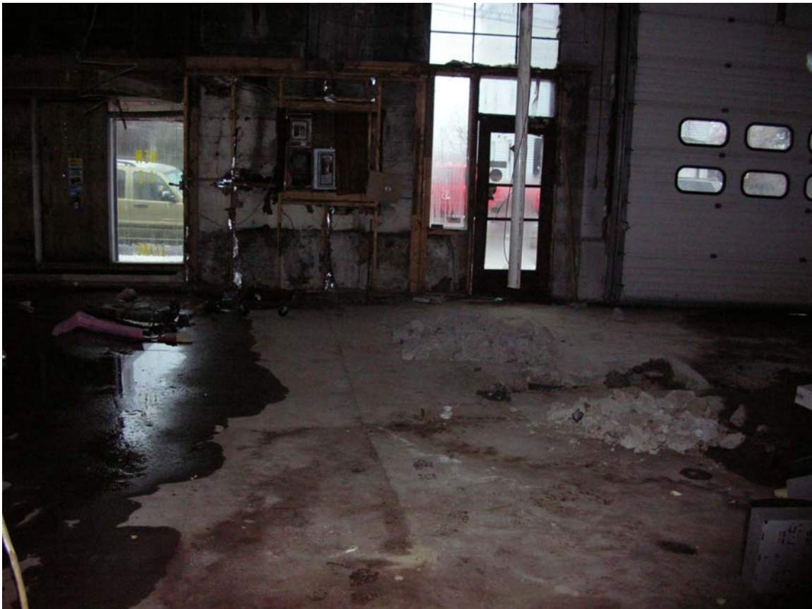
Photo 2: Front interior of building with sewer opening in floor
