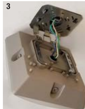
Complete wiring connections.
